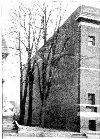
ILLUSTRATION 20. BLANK WALL OF PARISH HOUSE, FIRST BAPTIST CHURCH. THIS PREVENTS ADEQUATE LIGHTING OF LARGE ROOMS
