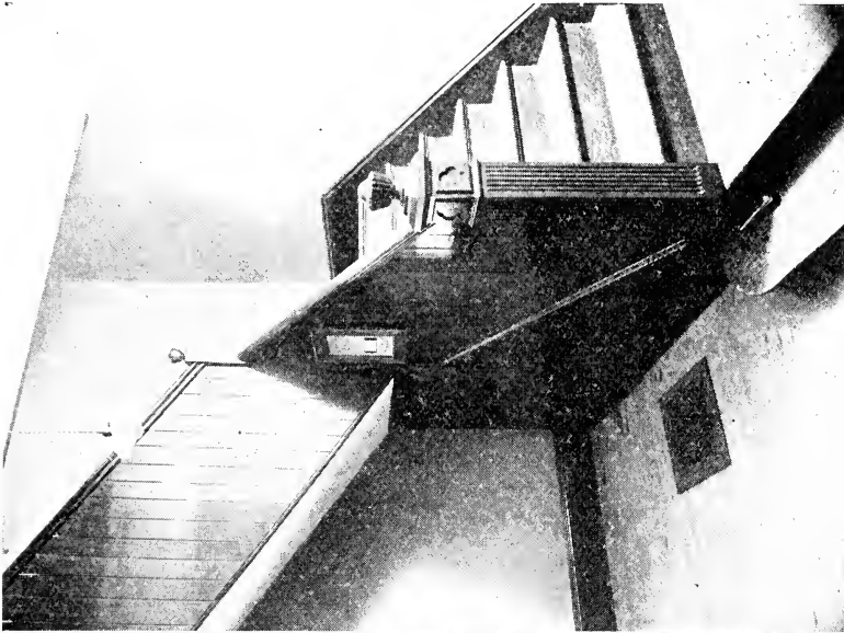
ILLUSTRATION 34. THE UNPROTECTED FRONT STAIRWAY LEADING FROM THE AUDITORIUM SHOWN ON OPPOSITE PAGE
