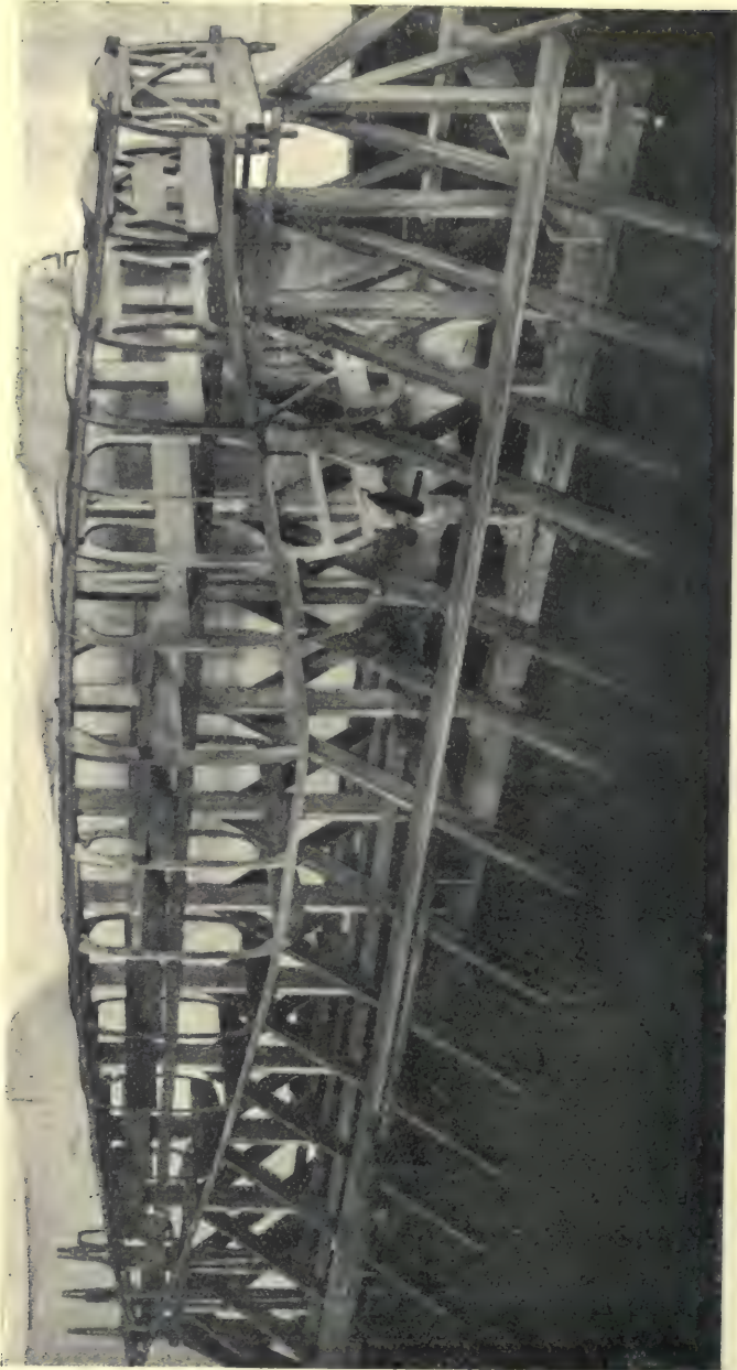
FIG. 14.—BULKHEADS AND LONGERONS OF VENEER FUSELAGE ASSEMBLED ON JIG READY FOR APPLICATION OF SKIN.
