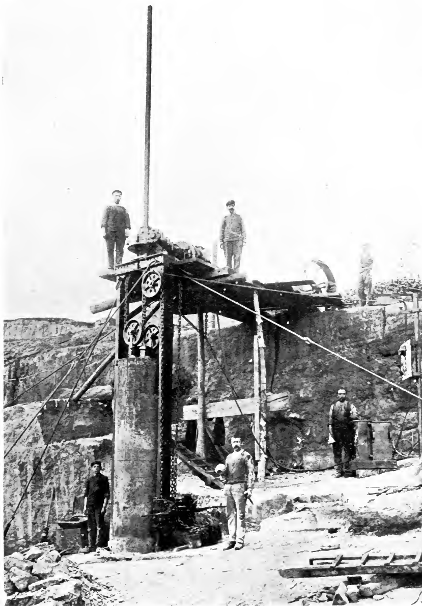
PERFORATING DRILL FOR SINKING HOLES FOR WIRE SAW. Lifting out the marble core.
