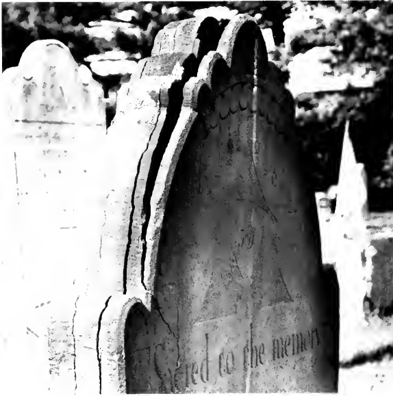
Bedminster, N.J. Cracks develop and widen, then stone layers pull apart during the initial phase of eradication caused by the freeze/thaw cycle.
