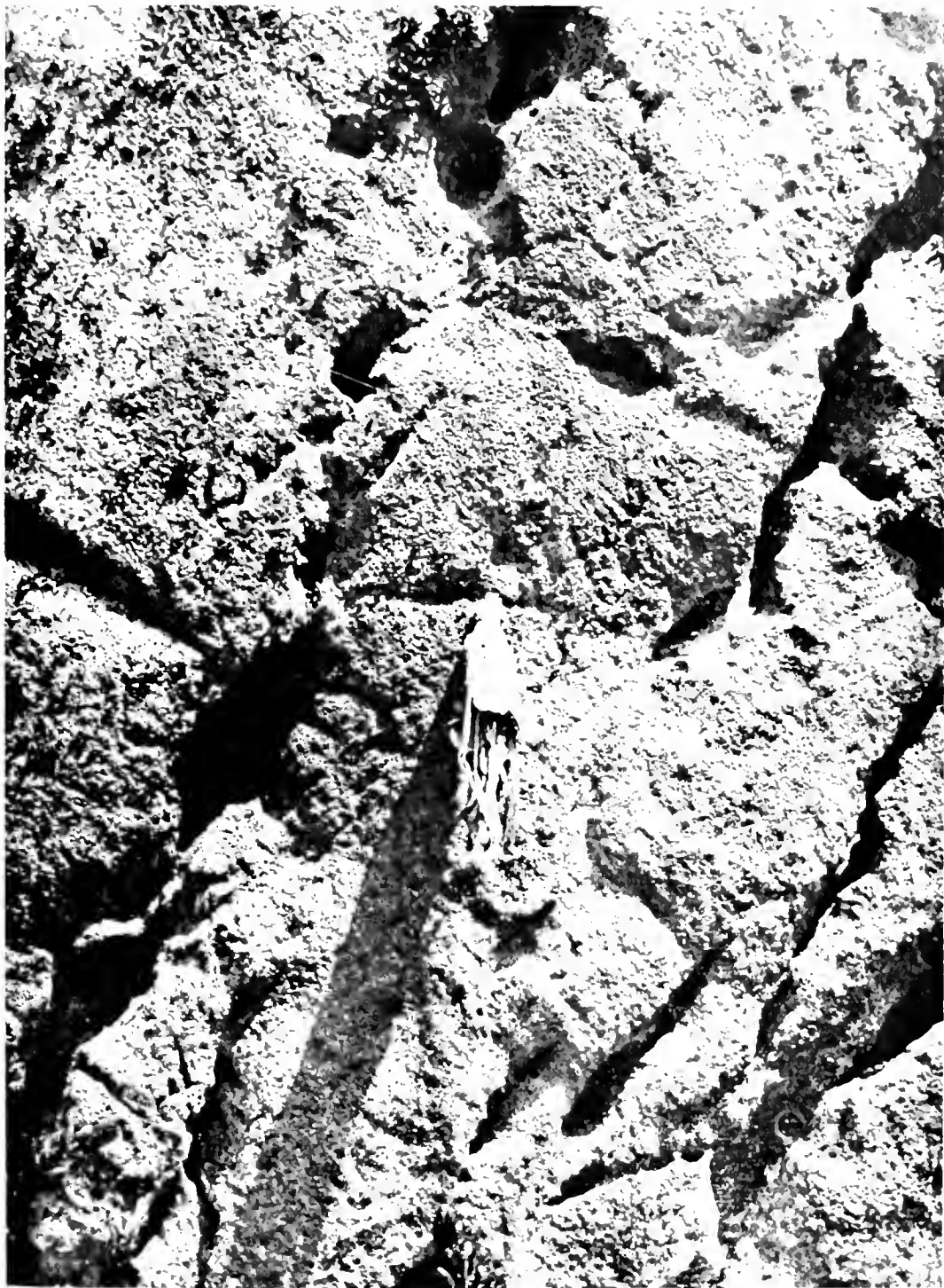
Fig. 1. A large, dark, vertical crack or crevice running down the center-left of the rock face. The surface is highly irregular and porous, with many small pits and larger, deep shadows. The lighting is harsh, creating deep shadows and bright highlights, emphasizing the rough texture.
