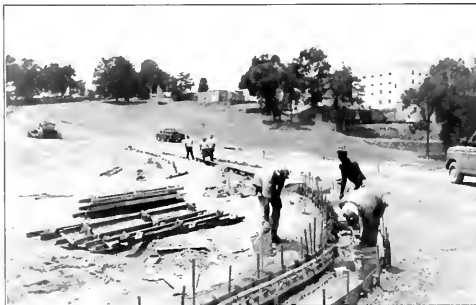
Construction of the Coalter Street entrance after MBC purchased the former SMA campus.
