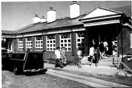
Pannill under construction and soon to be a hub of student-centered activities
