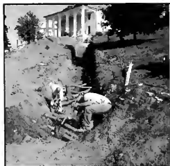
6/20/06 – Workers remove pieces of an old steam line inside a massive trench stretching from behind Carpenter Academic Building toward Miller Chapel
