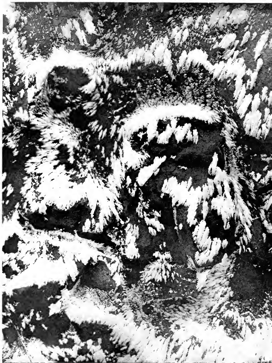
FROST FIGURES FORMED ON STONE COLUMN OF MT. WEATHER OBSERVATORY BUILDING, DURING ICE-STORM OF MARCH, 1906.
