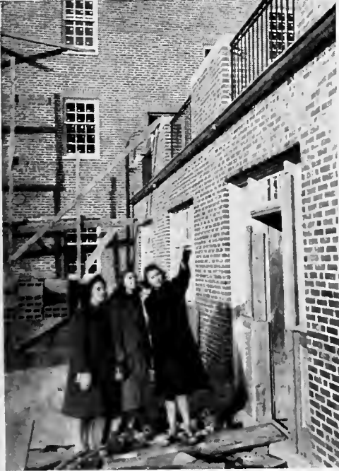
CO-EDS EXAMINE CONSTRUCTION WORK AT NEW DORMITORY LEFT TO RIGHT: MARJORIE ALDRICH '43 OF SPRINGFIELD, GLADYS FISH '41 OF PITTSFIELD, MARION AVERY '42 OF POCASSET.
