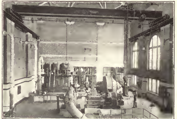
20-Ton Crane in a Pumping Plant.
