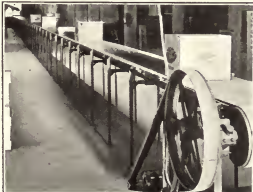
200' c. to c. 30" Belt distributing cases in warehouse of well known paper manufacturer.
