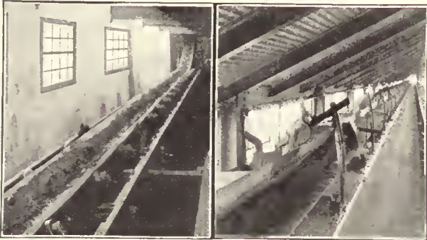
Belt Conveyor Carrying Coal. Belt Conveyor Carrying Sand.
