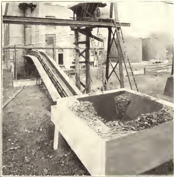
Conveying Coal from Hopper to Power House.
