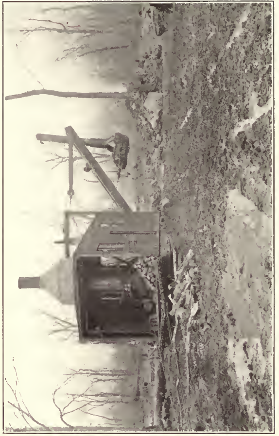
Skid-Derrick Type Steam Power Shovel Equipped with Drag-Scoop, Excavation Work in Marshy Land
