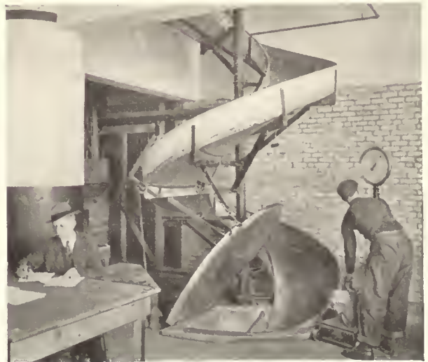
This Lamson spiral chute carries products from a number of floors to a delivery point on first floor. Note hinged fire door which also serves as deflector when goods are delivered at intermediate floors. Army Base Warehouse, Boston, Mass.
