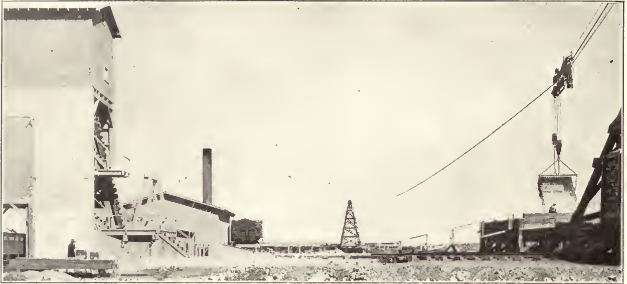
Endless-Rope Suspension Cableway Handling Loose Material with a Skip
