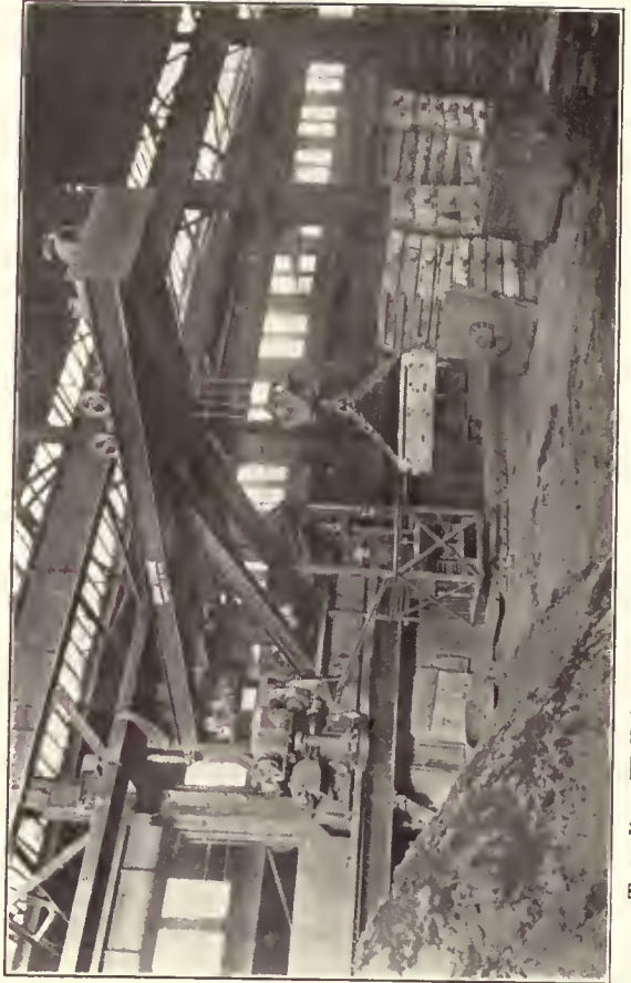
Traveling Wall Jib Crane Installed in a Foundry for Handling Molds
