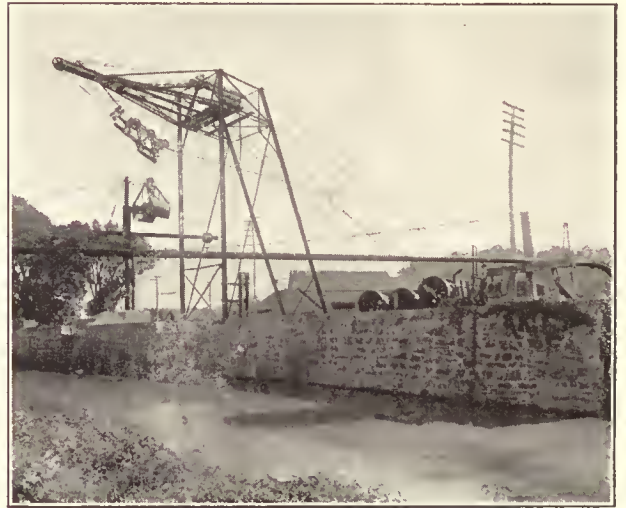
Head Tower with Projecting Boom
