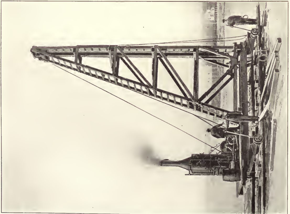
Movable Steam-Operated Pile Driver Derrick, Mounted on Rollers and Traveling on Wooden Runway
