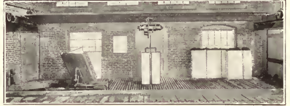
Maris Hand Push Crane with Enclosed Electric Hoist in Can Ice Plant.
