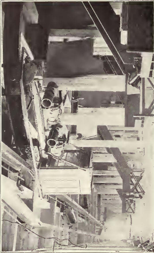
Double-Hook Electric Monorail Hoist, Installed to Handle Material Delivered by Chute from Upper Floor
