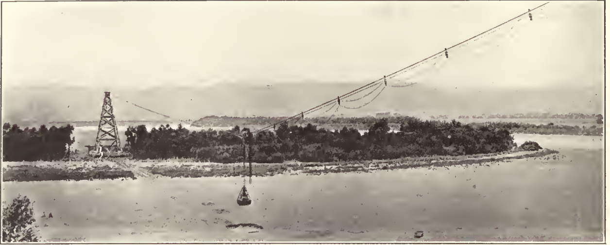
Suspension Cableway Dredging Sand from the Bed of a River and Delivering to a Bin for Drying
