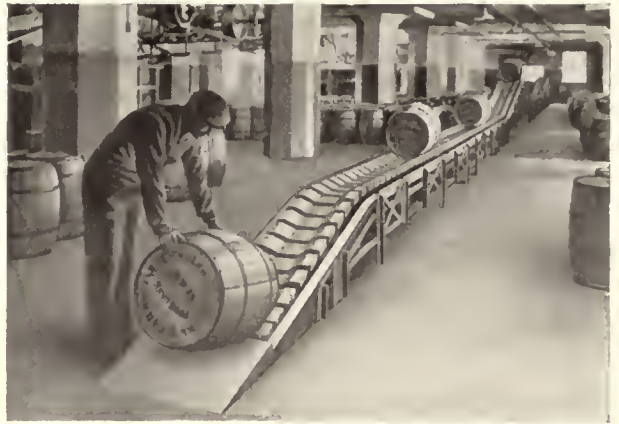
Lamson heavy duty slat conveyors are built in different types to carry barrels, cases, castings, bales, and other heavy loads. Revere Sugar Refinery, Charlestown, Mass.
