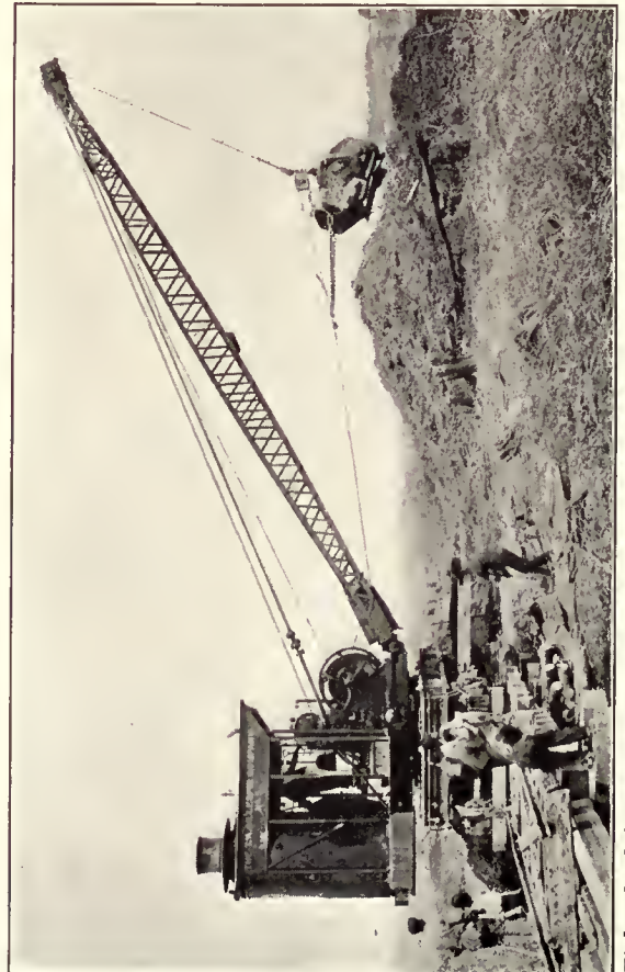
Eight-wheel Steam Locomotive Crane Handling Dragline Bucket in Excavation Work. Side Outriggers in Place
