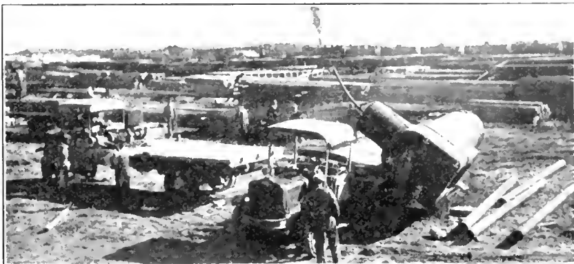
The White winch which may be had on 2, 3-3/4 or 5-ton models saves time and man-power in handling materials which have both bulk and weight. Above, an oil field boiler is being loaded upon a 5-Ton White with platform body.
