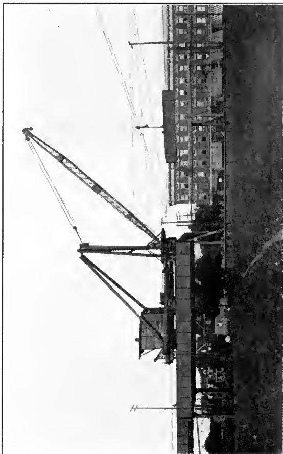
Traveling-Car Stiff-Leg Derrick Handling Girders in Elevated Railroad Construction Work. Wooden Frame, Steel Boom
