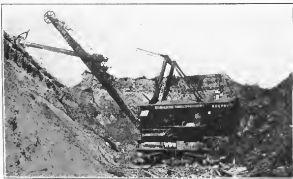
Electric Shovel Digging Power Canal at Niagara Falls, Canada, Operated by A. C. Type MA Motors.
