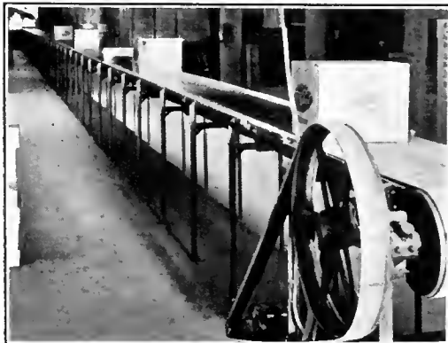
200' c. to c. 30" Belt distributing cases in warehouse of well known paper manufacturer.
