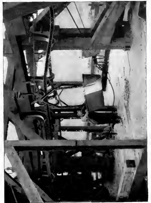
Loading Terminal Showing Carrier with Overhead Grip Passing Down Inclined Rail to Attaching Point
