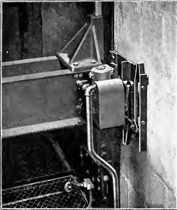
Leveling Switch on Top of Car and Cams in Hatchway, Micro Leveling Elevator.
