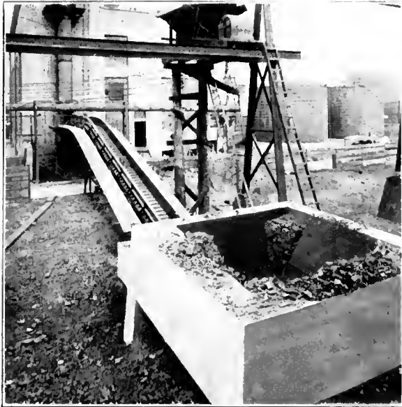
Conveying Coal from Hopper to Power House.
