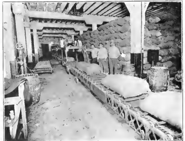
Floor Type Conveyor Installed, Showing Three Power Units.
