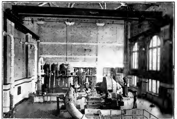
20-Ton Crane in a Pumping Plant.
