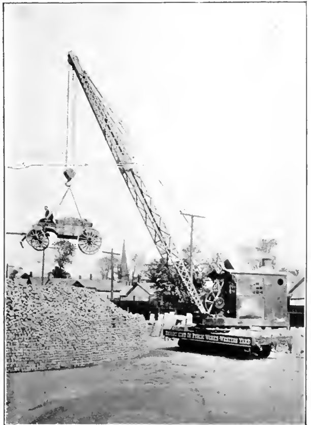
Steam Locomotive Crane Handling Paving Blocks in Dump Wagon with Fall Block, Hoisting Hook, and Chain Grab Hooks
