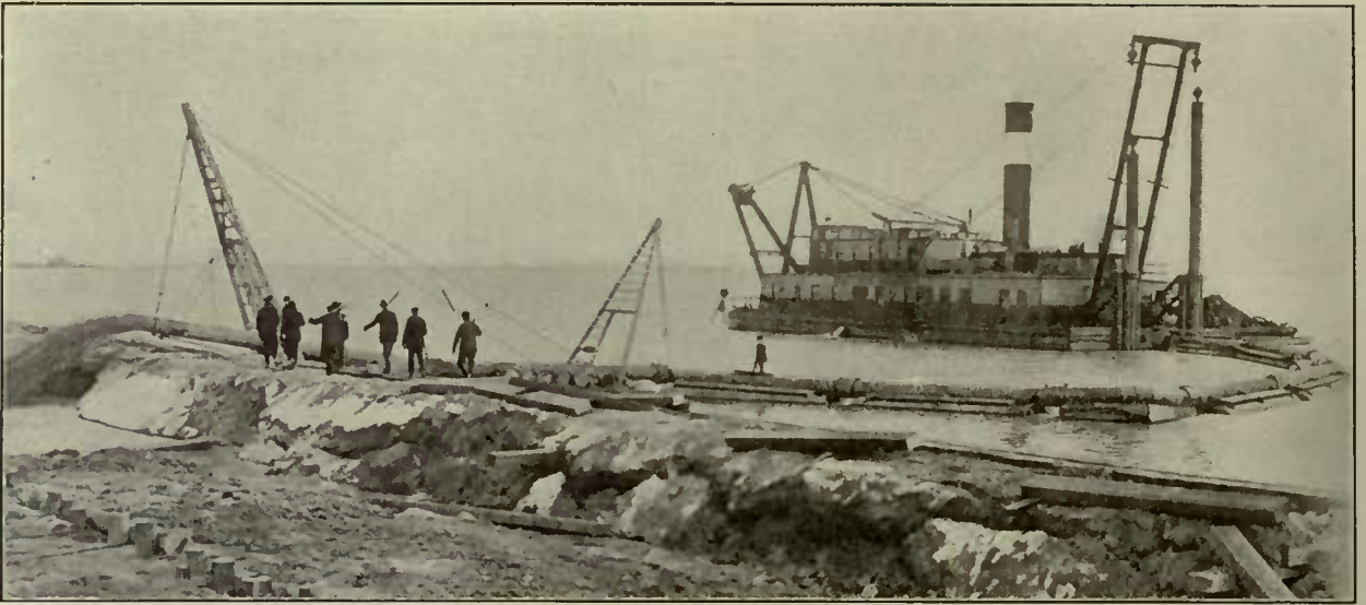
Hydraulic Dredge with Vertical Spuds. Disposal Pipe Line Laid for Filling Behind Bulkhead
