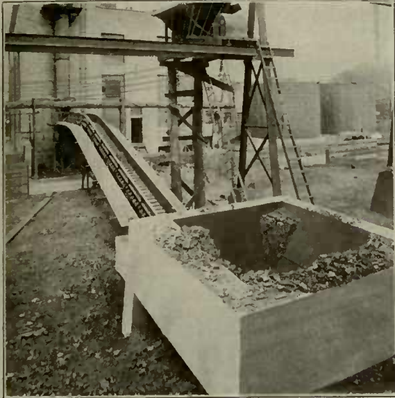
Conveying Coal from Hopper to Power House.
