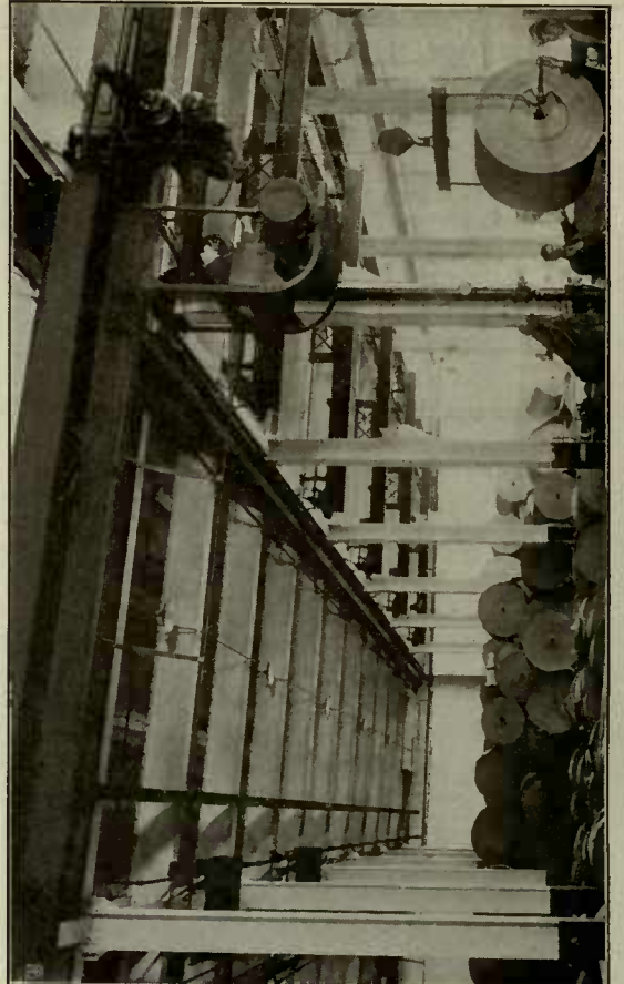
Electric Monorail Hoist Handling Rolls of Paper
