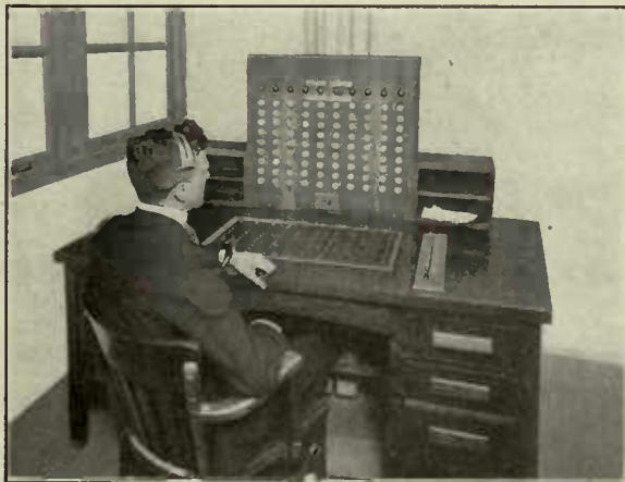
Central Dispatch Board for a group of ten elevators—United States Army Base, Brooklyn.
