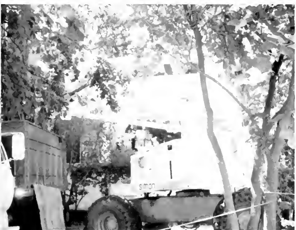
Large construction vehicles cluttered the campus over the summer as one of the largest renovation projects in years was undertaken.
