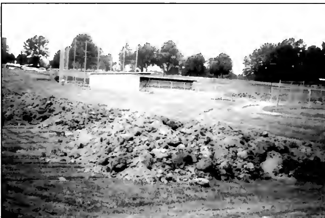
Right in step with other construction sites the ground is broke for the new Intramural field
