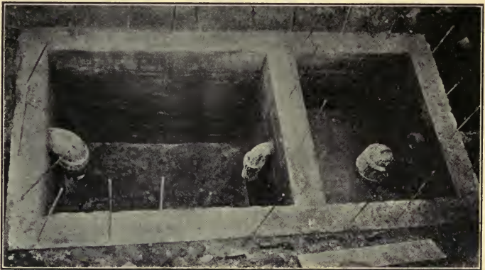
FIG. 156a—Photographic reproduction of a concrete septic tank, similar to that of Fig. 153. The tank requires only the cover to make it complete.
