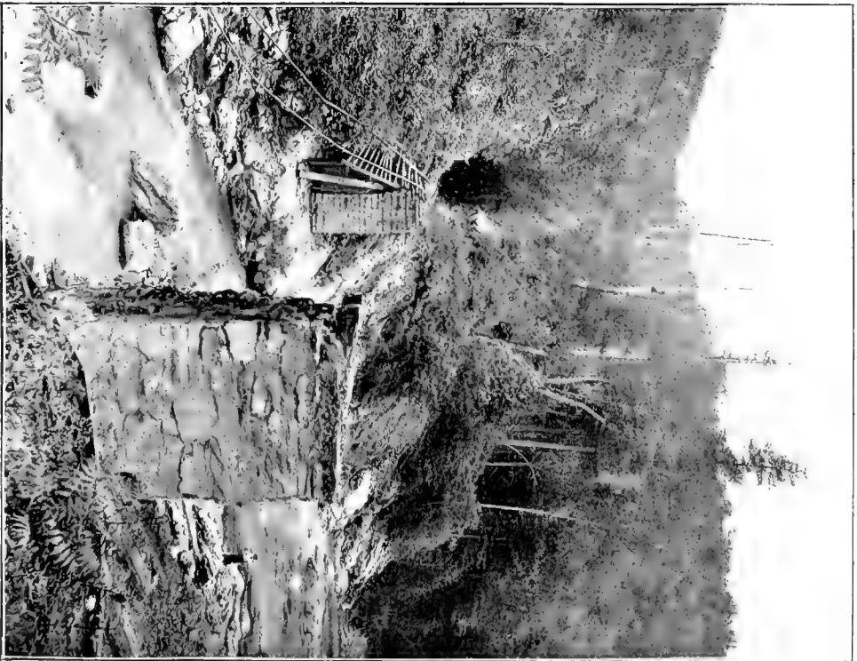
(B) FLOOD DAMAGES TO RAILWAY ON NOLCHUCKY RIVER, EAST TENNESSEE.
