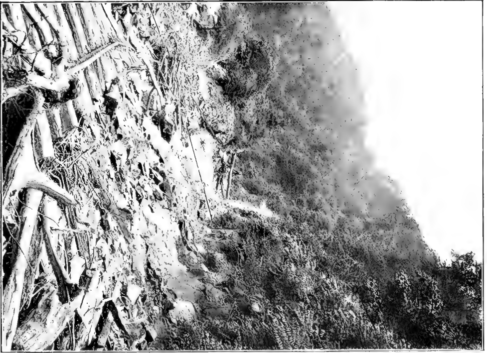
(A) FLOOD DAMAGES TO RAILWAY ON DOE RIVER, TENNESSEE. (See Pl. 82, 130.)
