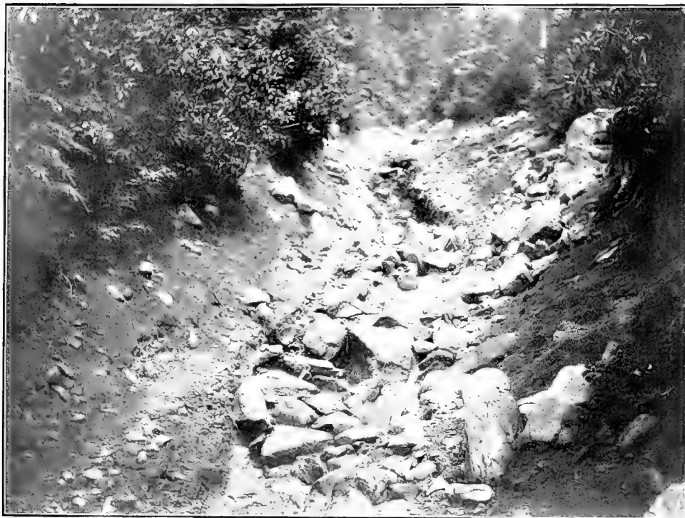
(B) PUBLIC ROAD RUINED BY FLOODS, MITCHELL COUNTY, N. C.
