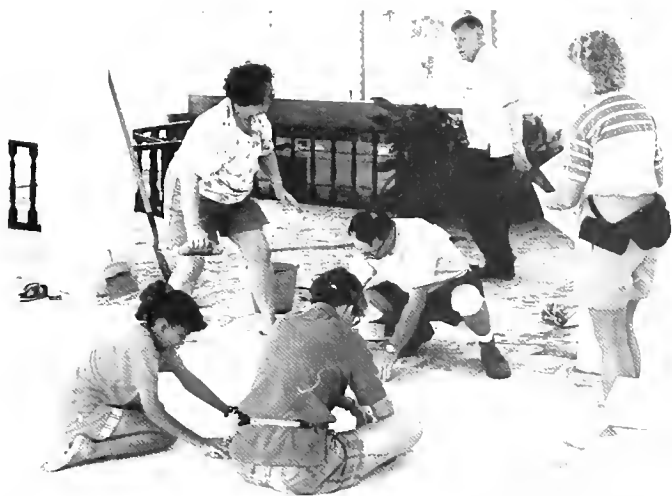
Among the projects of Bremen Brethren in Puerto Rico was installing a tile floor in the Caimito church sanctuary.
