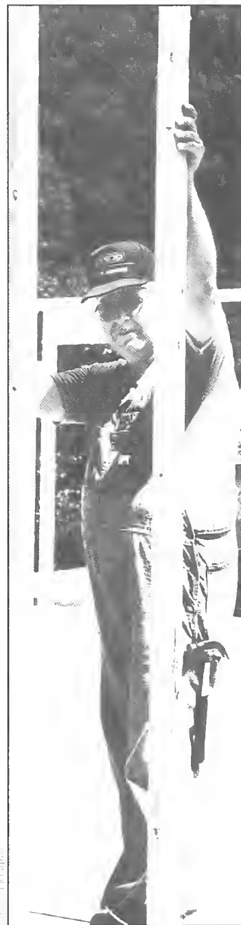
Putting his faith into action, Fred Bernhard works on a building project in Kentucky.
