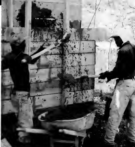
Workers mix and pour concrete in the forms to make the six-inch-thick walls.
