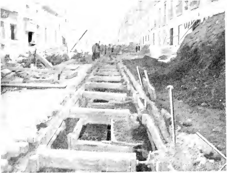
Drainage excavations, Escaderillas Street, in which over ten tons of Aztec treasures were found.
