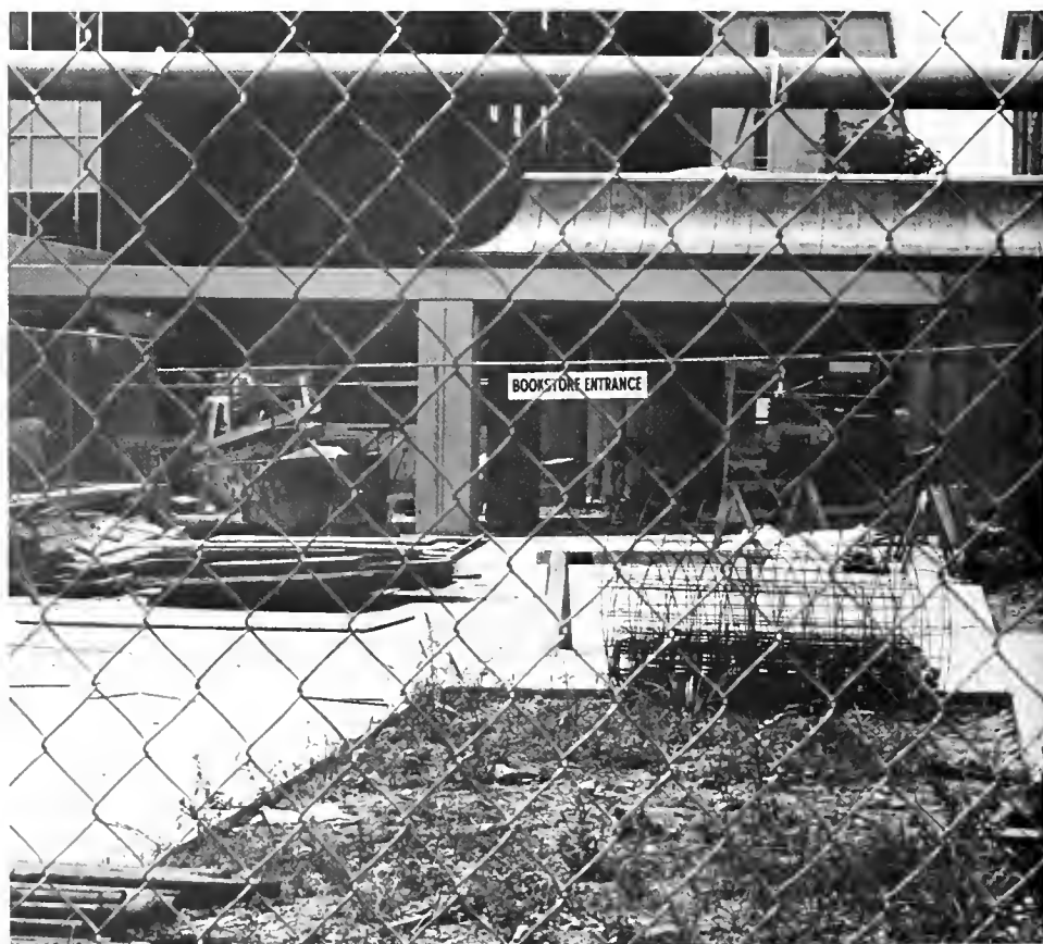
Fences enclose the University store and Jane F. Campbell Building during construction.
