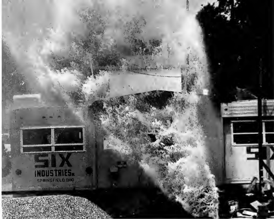
A ruptured water main delays construction on the Jane F. Campbell Building. Right: Construction workers stand idle awaiting repair of the broken water main.
