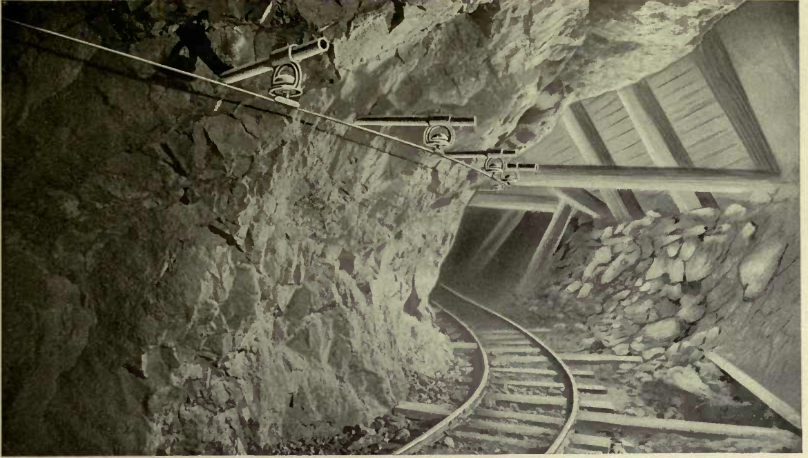
Method of Attaching Trolley Directly to Side Wall (Using Form "D" Suspension)
