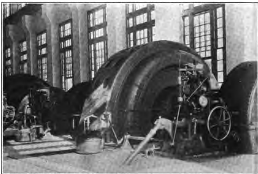
Photo No. 69. Generators and water wheels, No. 1 power plant, Pacific Light and Power Company, Cascada, Fresno County.
