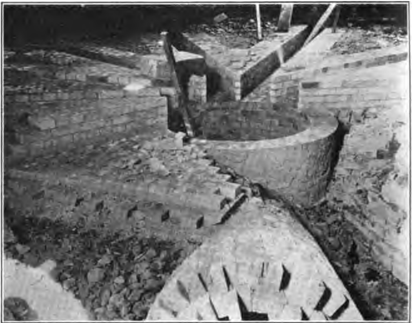
Floor construction of a brick kiln at the Carnegie Brick and Pottery Plant, San Joaquin County, California. Photo by Walter W. Bradley.
