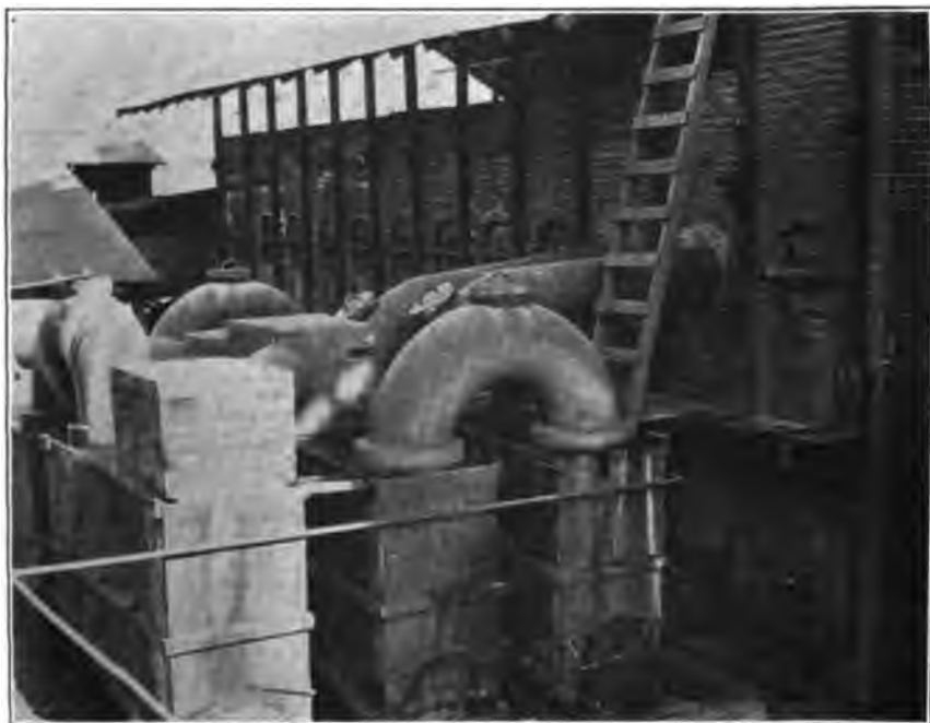
Photo No. 106. Condensers at Pacific Quicksilver Mine, Fresno County.
