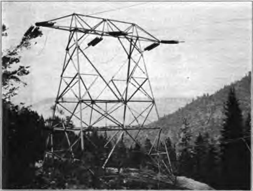
Photo No. 73. Transmission tower, 150,000 volts. Pacific Light and Power Company, near Cascada, Fresno County.
