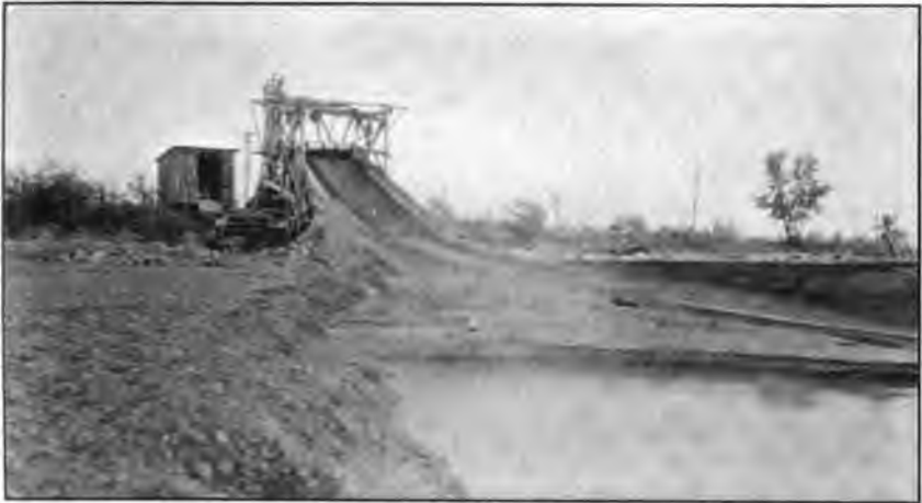
Photo No. 155. Drag-line excavator of Russian River Gravel Company, Healdsburg, Sonoma County, California.
