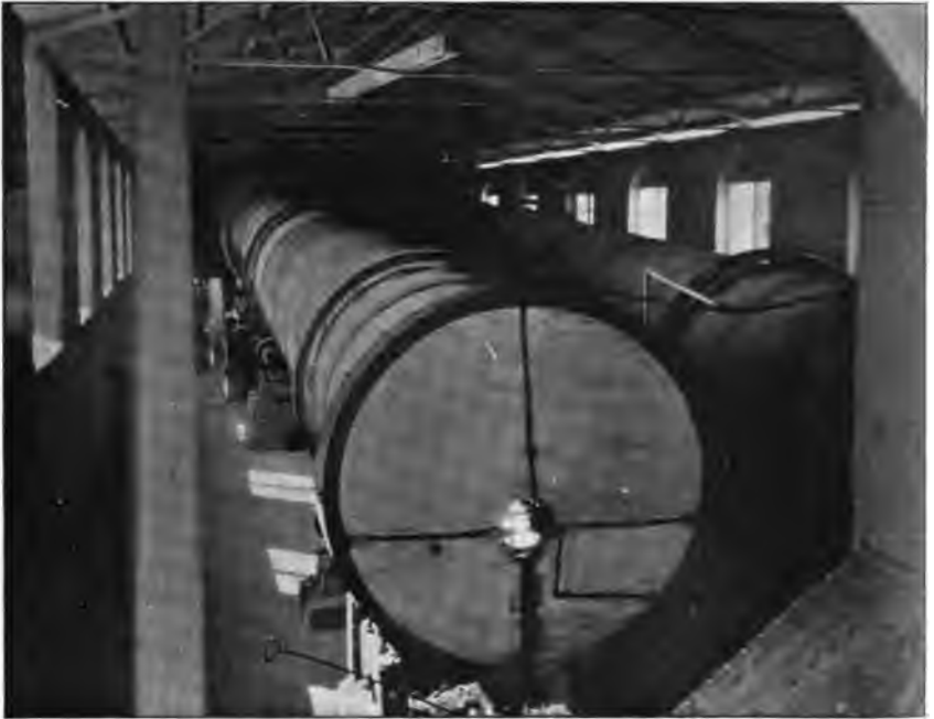
Photo No. 49. Rotary kilns in mill of Standard Portland Cement Company, Napa Junction, Napa County.
