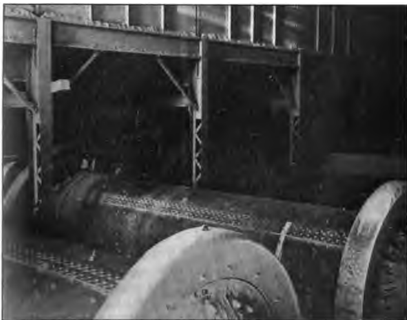
Photo No. 67. Tube mills and hoppers, for crushing raw materials in new mill of Pacific Portland Cement Company, Solano County.
