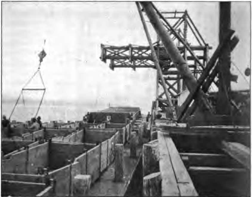
Photo No. 114. Daniel Contracting Company's loading pier and barges at San Pedro Point, Marin County, California.
