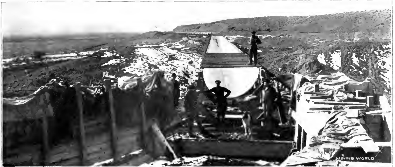
A 10,000-FT. METAL WATER FLUME IN COLORADO.
