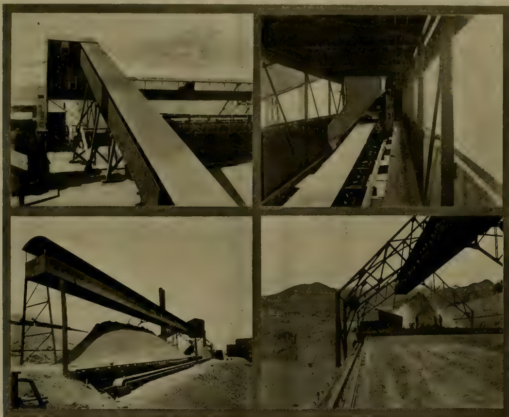
CONVEYOR LEADING TO BEDDING CONVEYOR. STACKING AND RECLAIMING CONVEYORS.
