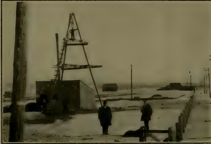
DIAMOND-DRILLING AT NEGAUNEE. THE LANDS WERE CONSIDERED VALUELESS FOR YEARS UNTIL DEEP DRILLING DISCLOSED LARGE OREBODIES.
