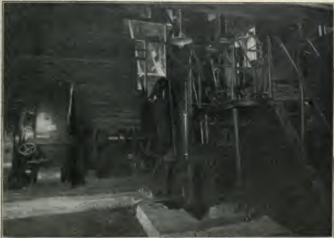
Fig. 3. Engine Room Showing Hoist in Place.
