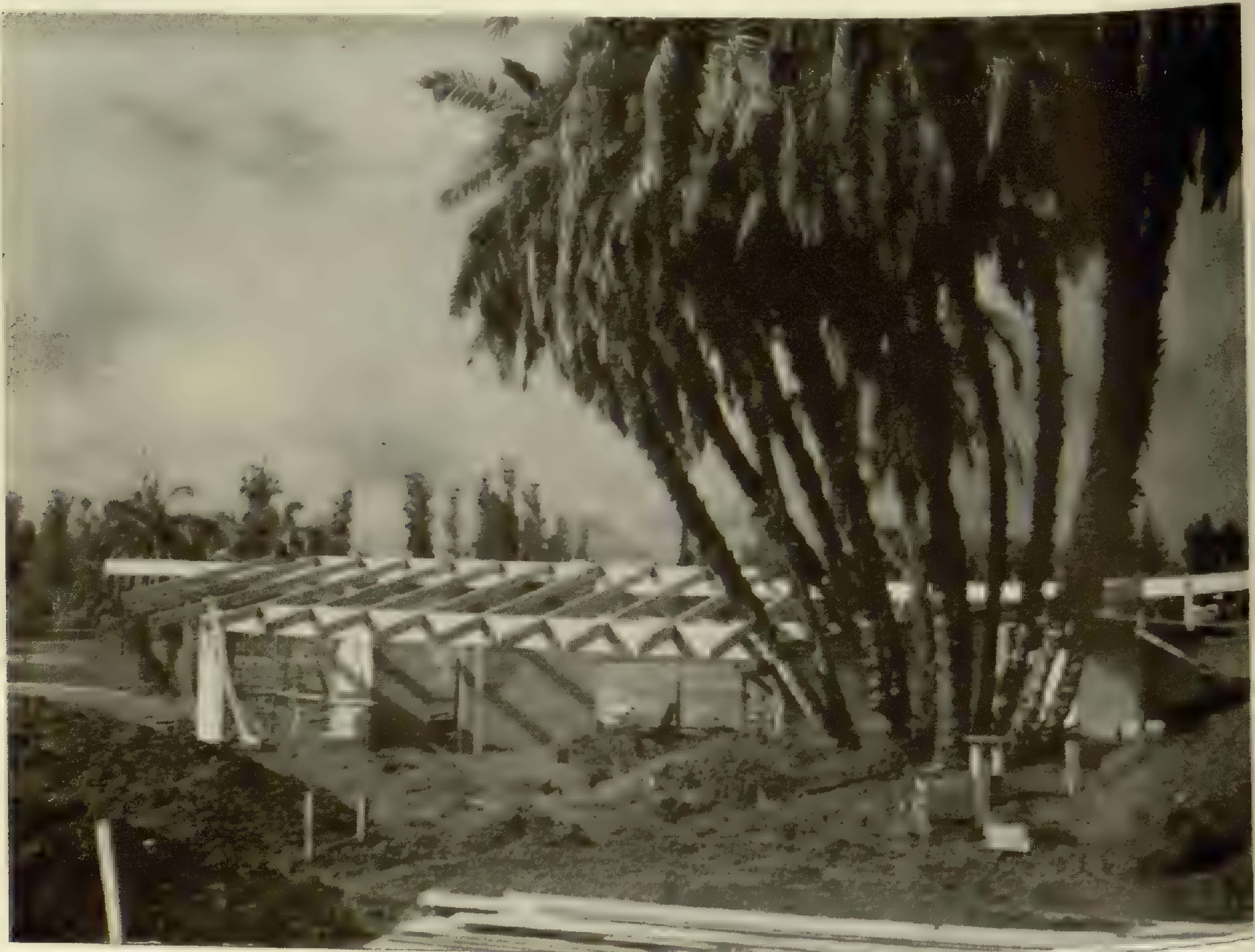
One can almost see our visitors passing through the turnstiles of the Arboretum's Gatehouse, at 301 N. Baldwin Ave., as the construction of this building and the Administration Building progress toward completion.
