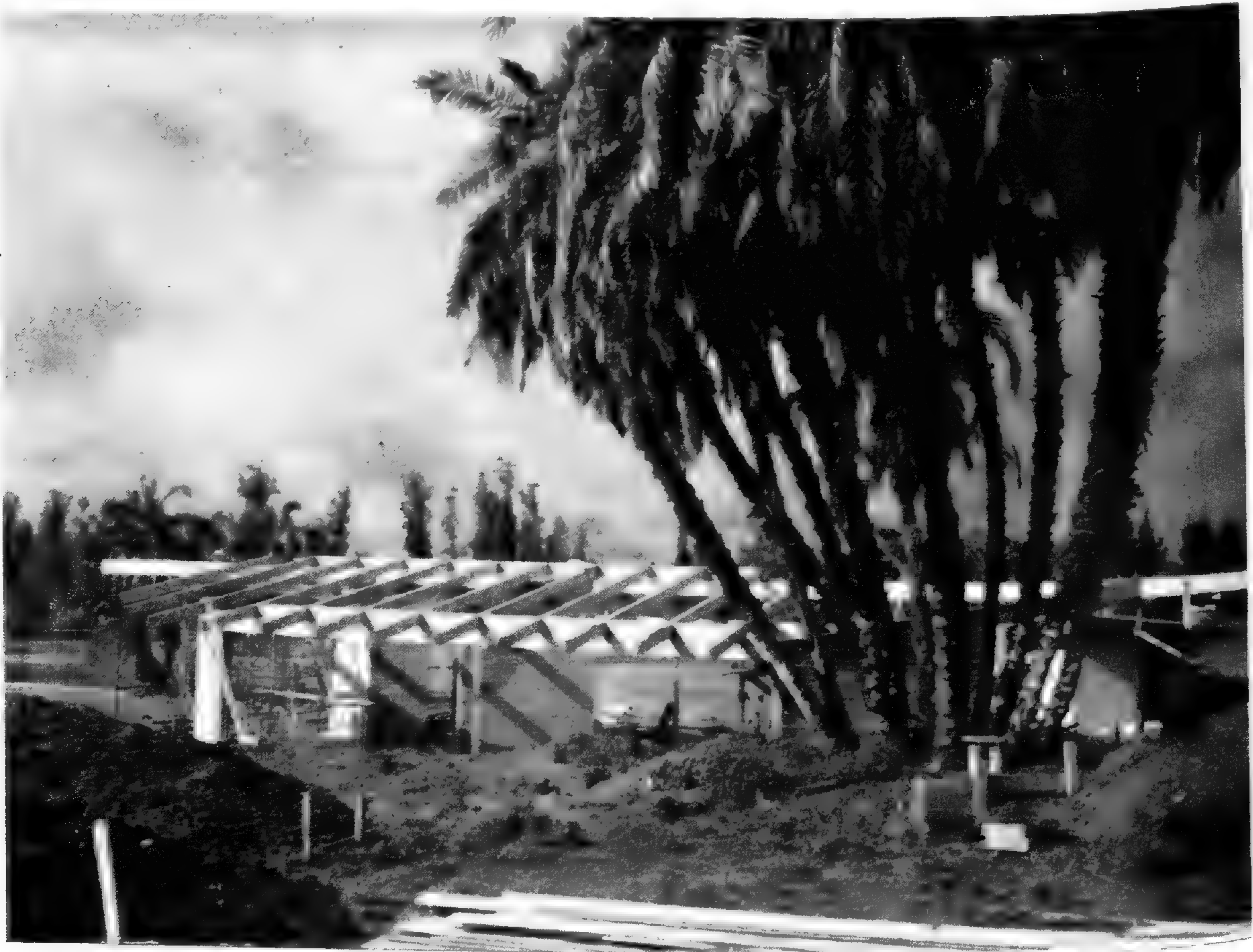
One can almost see our visitors passing through the turnstiles of the Arboretum's Gatehouse, at 301 N. Baldwin Ave., as the construction of this building and the Administration Building progress toward completion.
