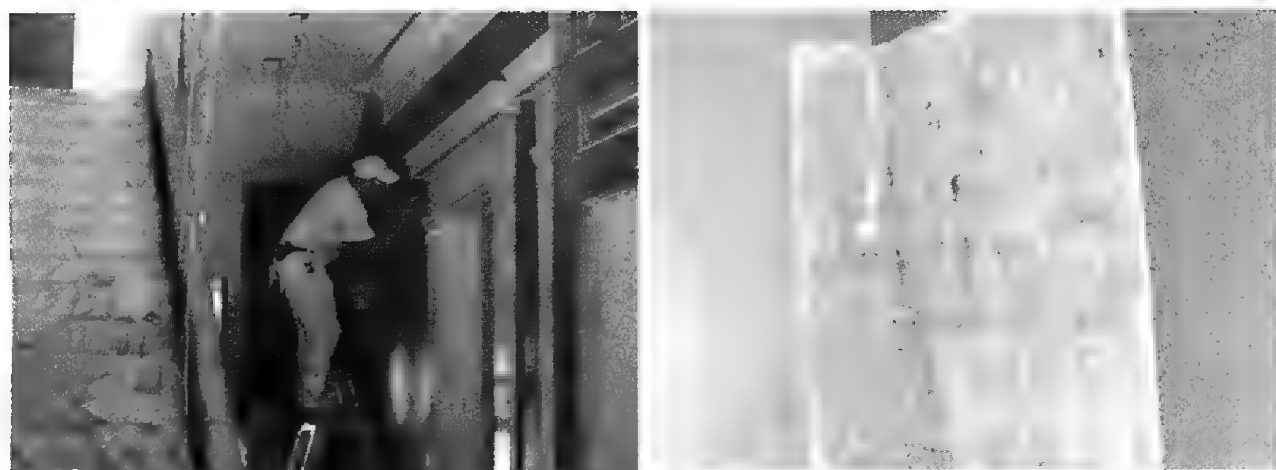
Renovation of Henry Shaw’s original country home, Tower Grove House, revealed surprises like the trompe-l’oeil paneling painted on a wall (lower right).
