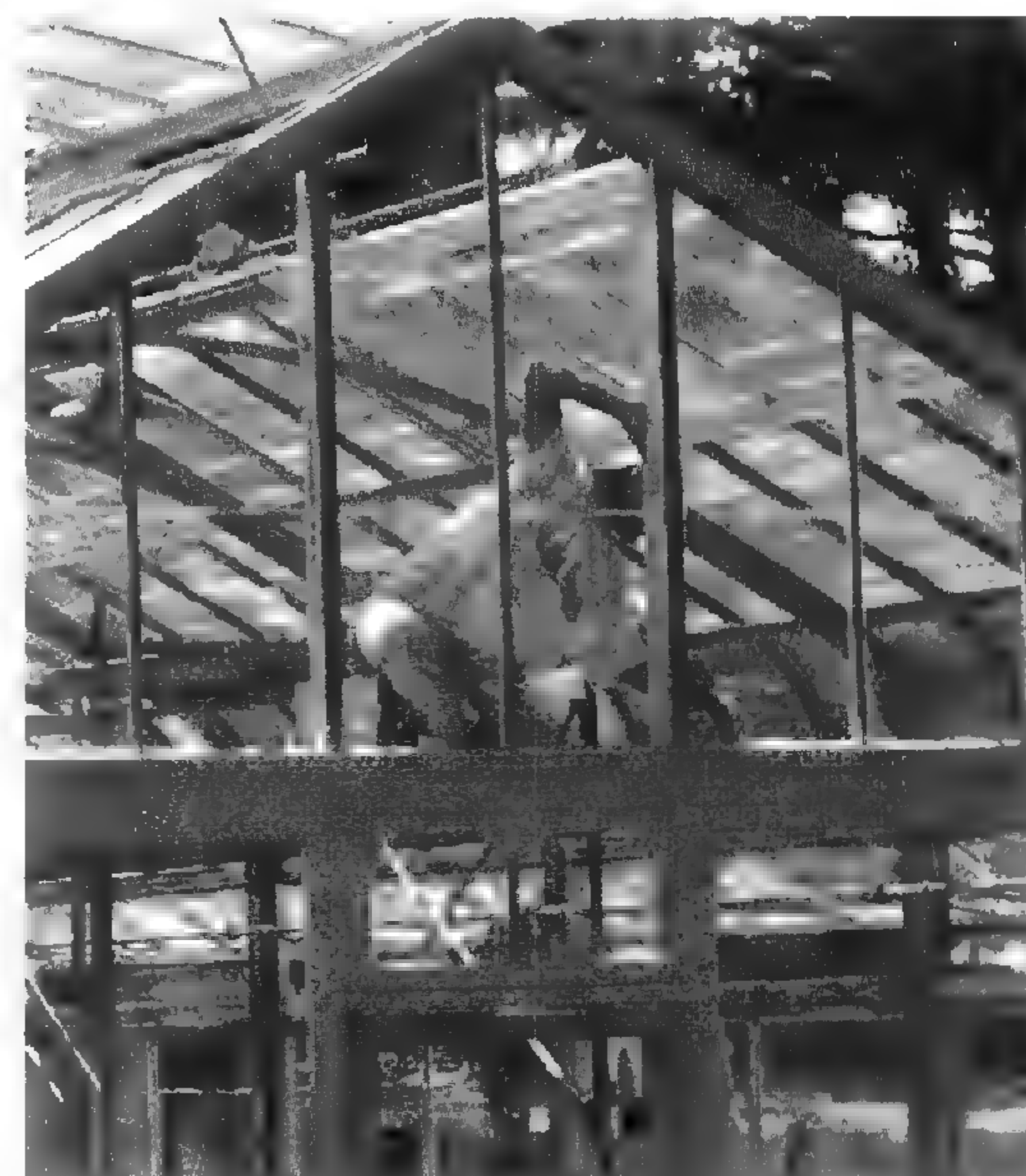
Greenhouse restored: The last remaining Faust family greenhouse in St. Louis County's Faust Park is being restored by the Butterfly House for use as a facility for quarantine and propagation of plant species housed in the Tropical Conservatory.
