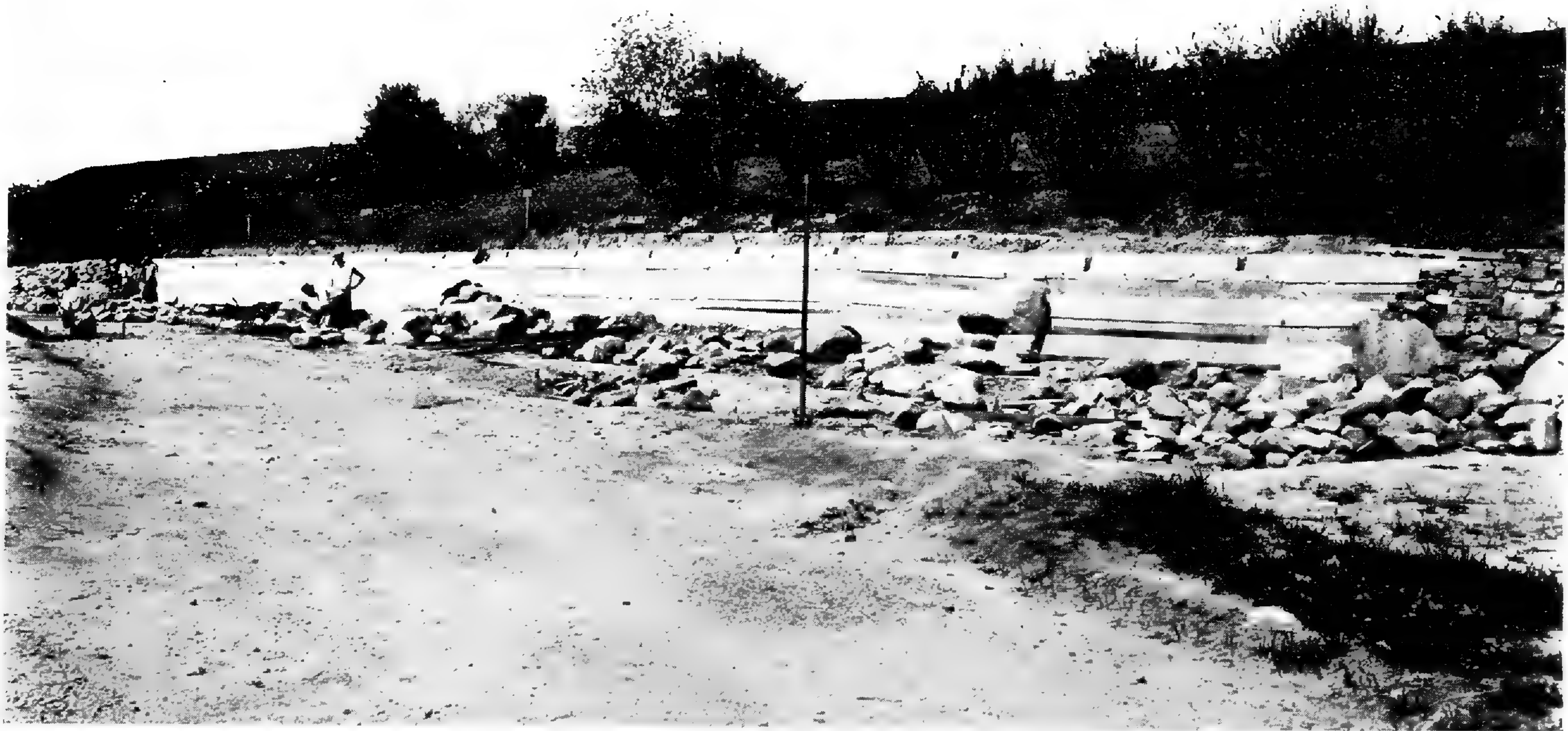
FIG. 2. North Addition development. Wall-garden wall against Reservoir embankment, showing reinforced concrete retaining wall against which the stone planting-wall is being built. Facing south-west. June 14, 1934. (8606)
