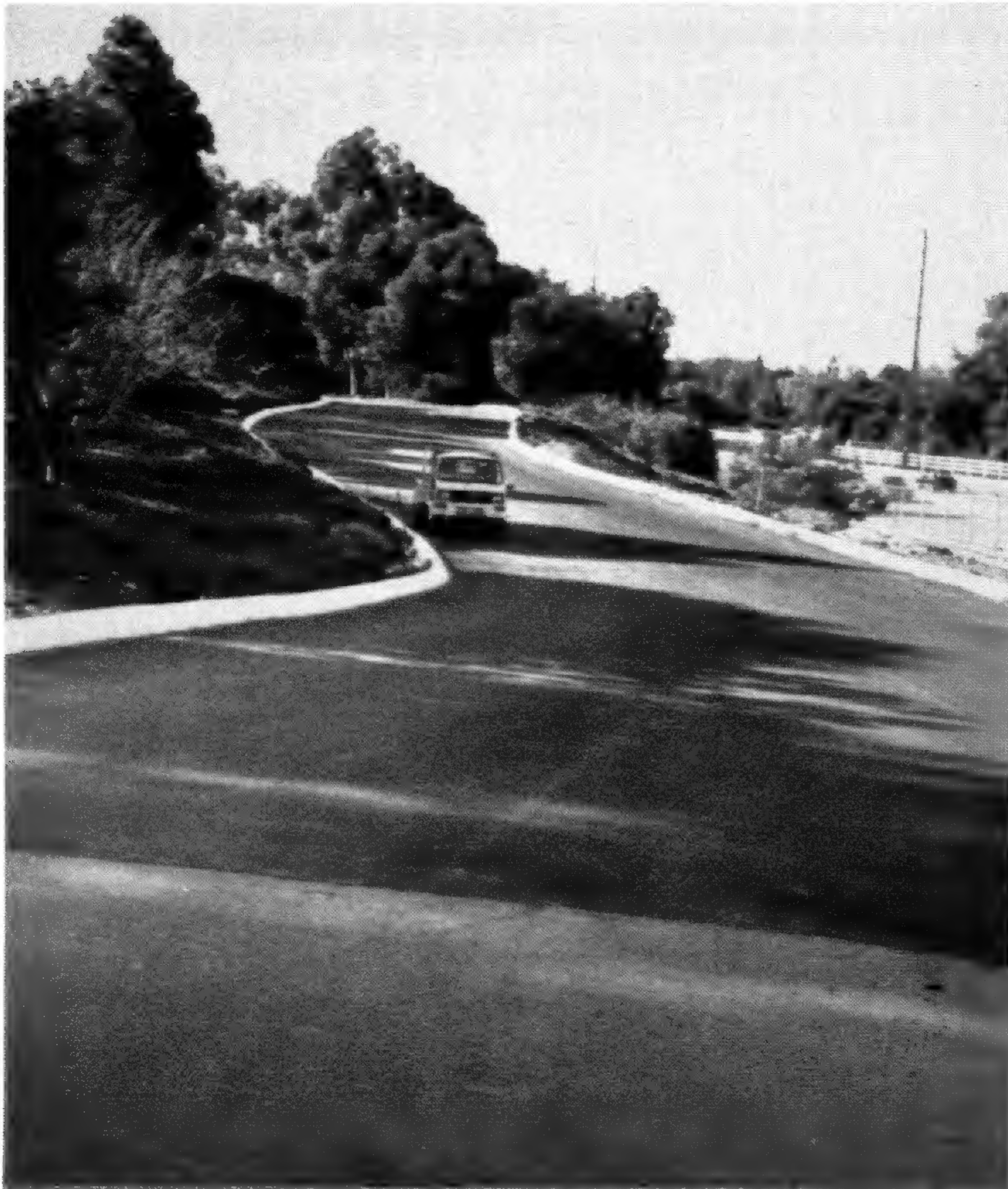
The entry road at South Coast is finished so work can begin on the next phase, new fences and signs.
