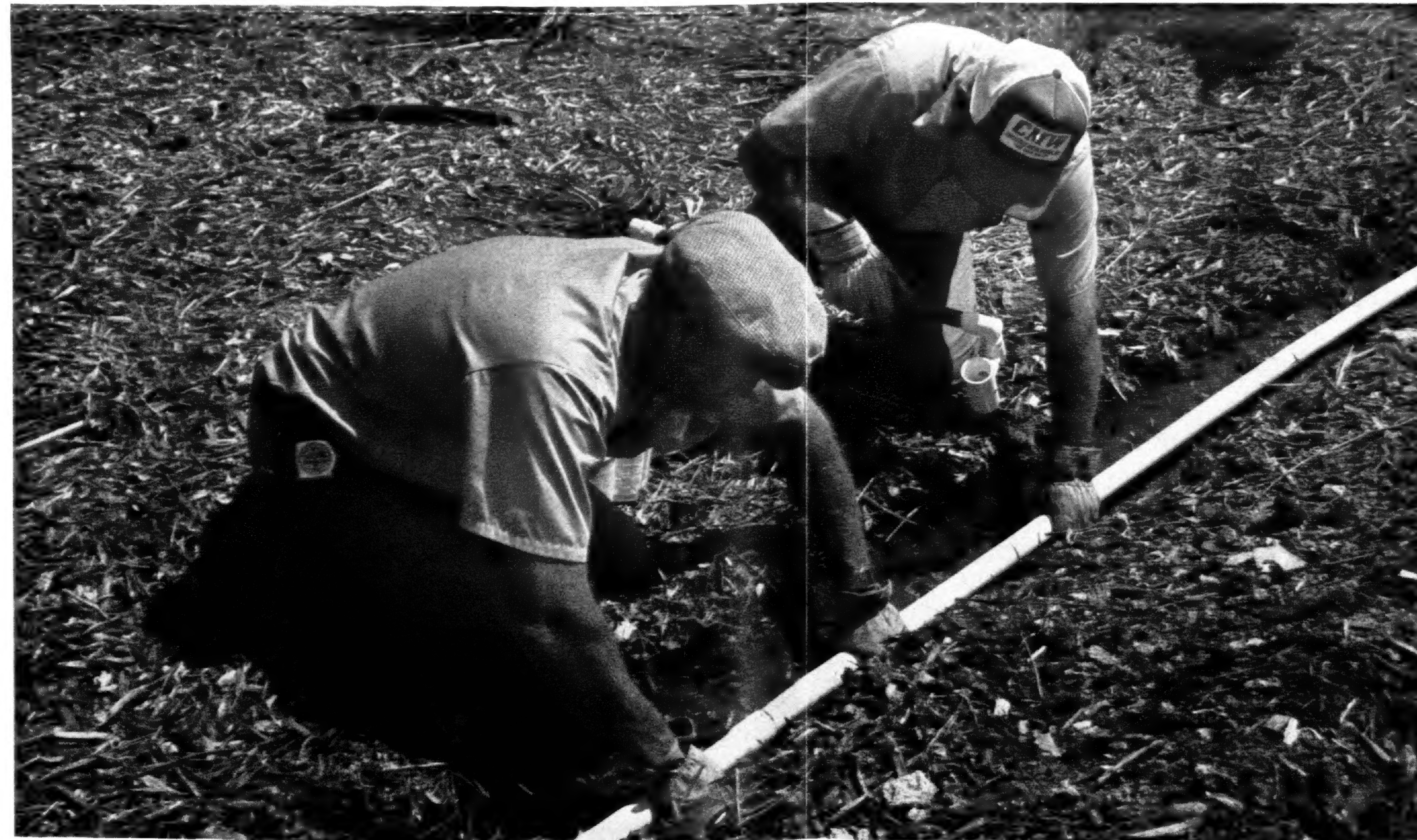
New irrigation lines being installed incorporate slip joints that allow pipes to move several inches without leaking.
