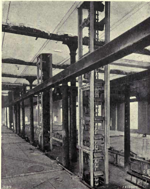
FIG. 73.—ELEVATORS FOR RAISING PURIFYING MATERIAL TO AN UPPER FLOOR AT THE NEEPSSEND GASWORKS, SHEFFIELD.
