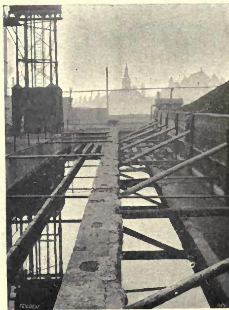
FIG. 35.—WATER CONDENSERS AT THE OLD KENT ROAD STATION, SOUTH METROPOLITAN GAS CO.
