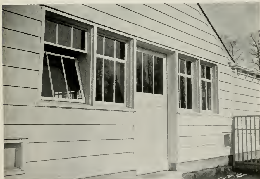
WINDOWS AS SHOWN BY THE DETAIL IN FIG. 22. FARM BUILDINGS FOR CLIFFORD V. BROKAW, ESQ., GLEN COVE, L. I.
