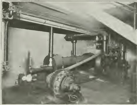
A motor driven compressor with brine cooler and brine pump.
