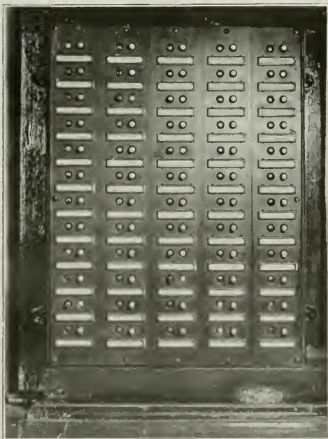
Fig. 1. The switchboard is located at the front desk in the main office.
