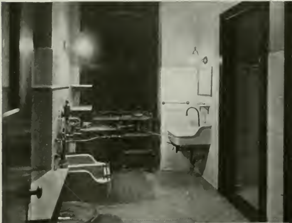
Fig. 8. Night view of a utility room showing the local lighting from bracket units over the sink and sterilizing apparatus. Sufficient light is transmitted through the opalescent reflectors to provide general illumination.
