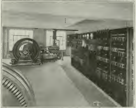
The switch board of the power plant.
