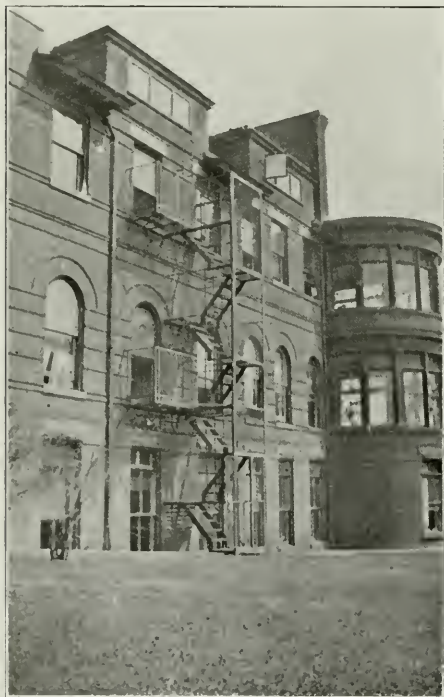
A hospital fire escape, fair as regards pitch of stairs and good as to screen enclosures, but containing so many 180° turns as to be useless for carrying down patients on stretchers.
