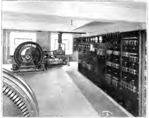
The switch board of the power plant
