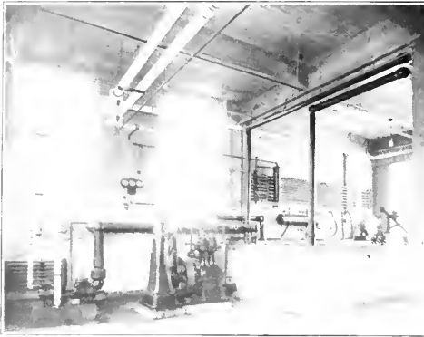
A compressor driven by a vertical steam engine. It operates refrigerators either by brine or direct expansion. It also operates the small ice making tank shown on the right.
