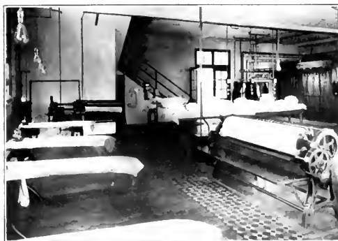
IRONING DEPARTMENT OF SMALL HOSPITAL LAUNDRY.
