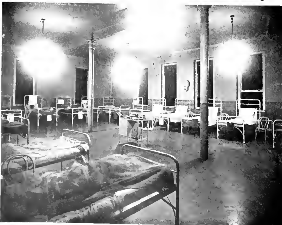
Fig. 6. Enclosing glassware which diffuses the light and which can be readily cleaned is used in this square-hopped ward for general illumination. Such lighting is simple of installation, inexpensive and a remarkable improvement over much of the equipment now in use.
