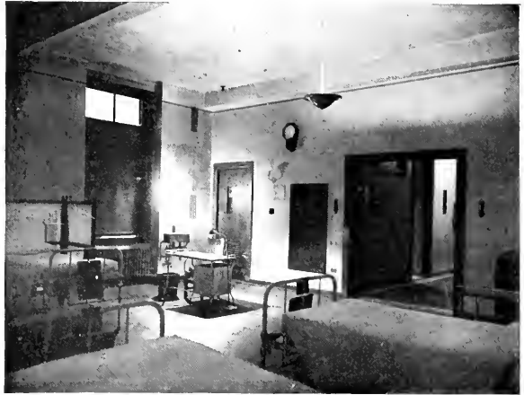
Fig. 7. A semi-private ward lighted by a single porcelain enameled totally indirect unit. The nurse's desk with a local light located near the main control panel will be noted. Baseboard receptacles and emergency lights are properly placed.
