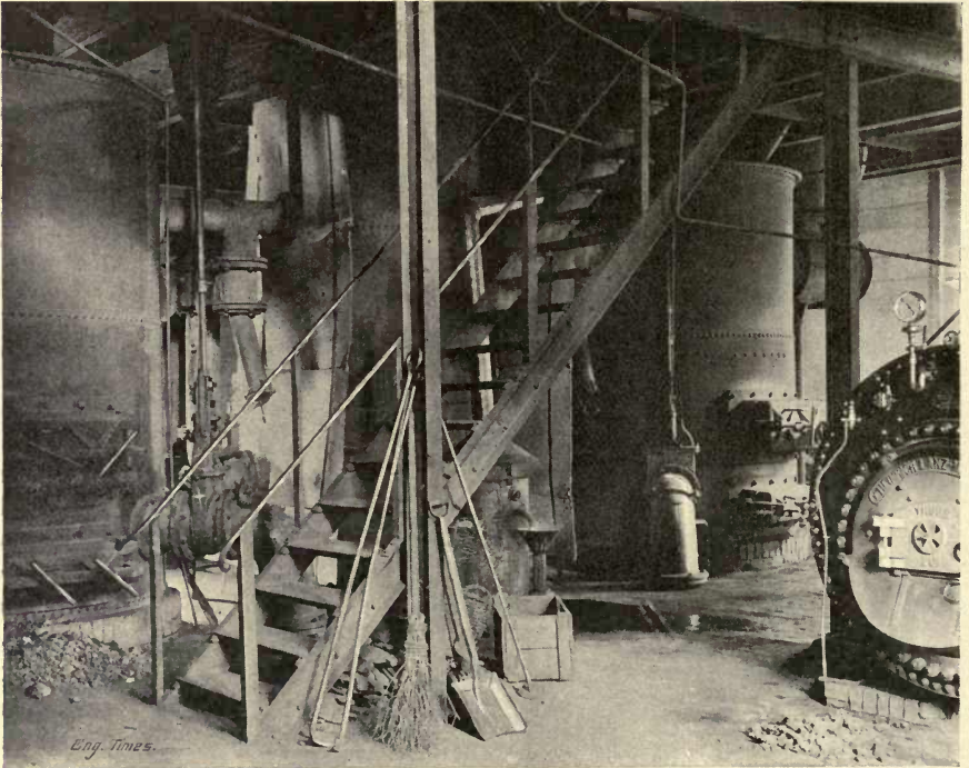
FIG. 47.—THE GENERATORS OF THE DELLWIK-FLEISCHER WATER GAS PLANT, KÖNIGSBERG.
