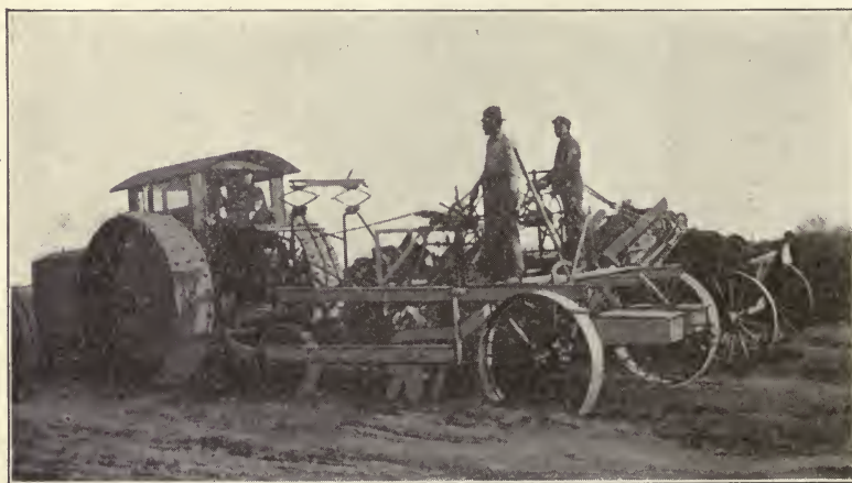
Fig. 54. Two Views of Elevating Graders Loading Earth into Dump Wagons Courtesy of Western Wheeled Scraper Company, Aurora, Illinois
