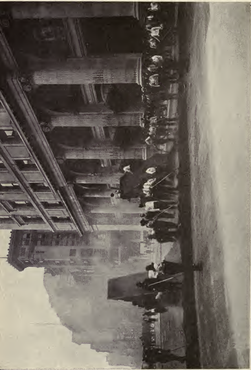
LAYING TRINIDAD SHEET ASPHALT PAVING IN FIFTH AVENUE, NEW YORK CITY Courtesy of Barber Asphalt Paving Company, Philadelphia, Pennsylvania
