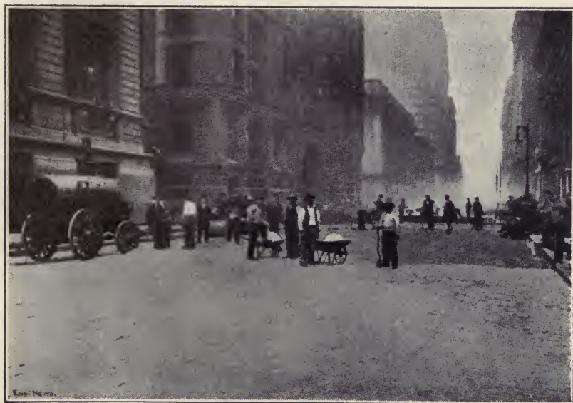
Fig. 95. Spreading Sand Filler on Wood-Block Pavement Courtesy of Engineering News, New York City
