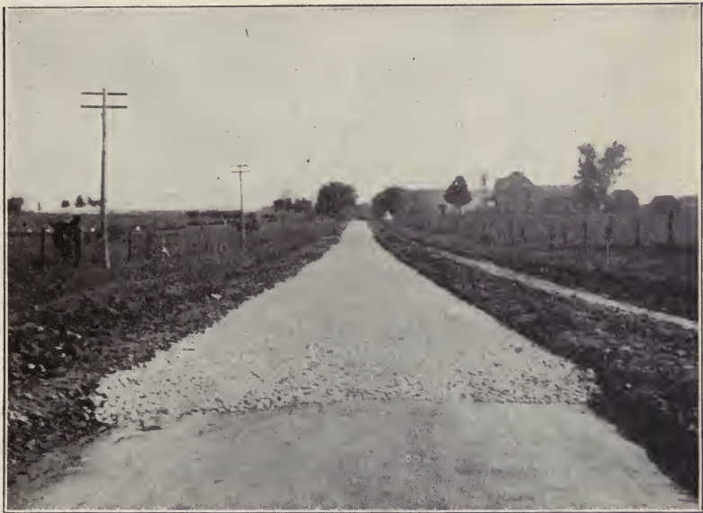
Fig. 62. View Showing Spreading of Lower Course of Macadam Road Courtesy of United States Department of Agriculture
