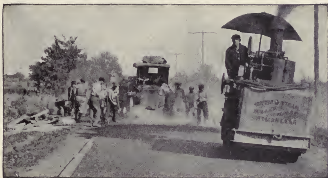
Fig. 68. Rolling Bituminous Macadam Road Surface Courtesy of Barrett Manufacturing Company, New York City
