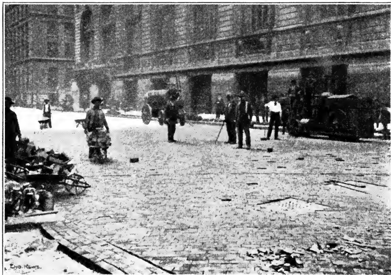
Fig. 94. Wood-Block Pavement Being Hammered and Rolled, Preparatory to Putting in Filler Courtesy of Engineering News, New York City
