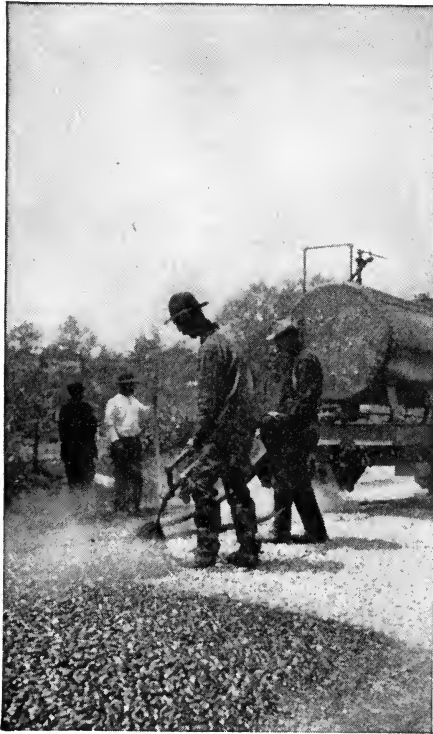
Fig. 65. Spreading Bituminous Binder by Pressure Nozzle, Penetration Method Courtesy of Barrett Manufacturing Company, New York City
