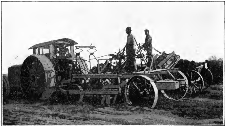
Fig. 54. Two Views of Elevating Graders Loading Earth into Dump Wagons Courtesy of Western Wheeled Scraper Company, Aurora, Illinois
