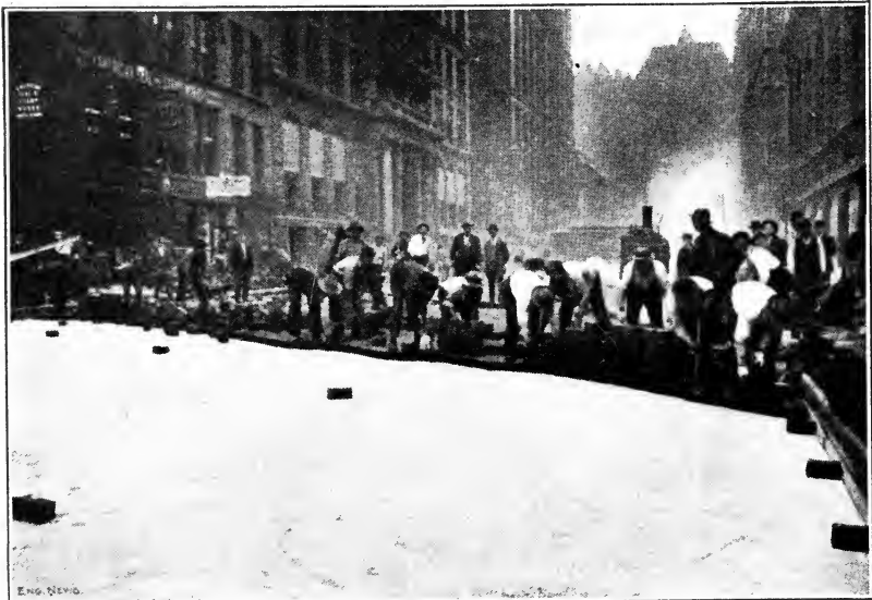
Fig. 93. Laying Wood Blocks in LaSalle Street, Chicago Courtesy of Engineering News, New York City
