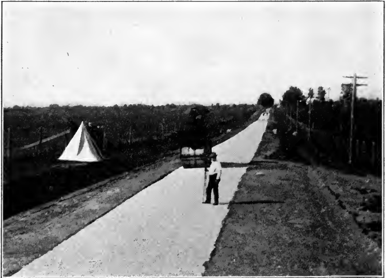
Fig. 63. Compacting Broken Stone by Steam Roller Courtesy of United States Department of Agriculture
