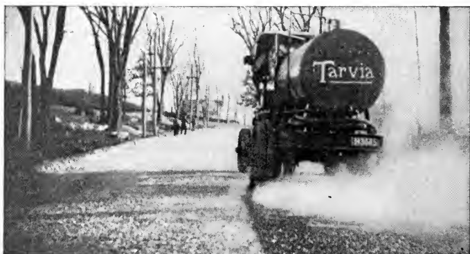
Fig. 69. Spraying Seal Coat by Auto Truck, One-Half Gallon to the Yard Courtesy of Barrett Manufacturing Company, New York City
