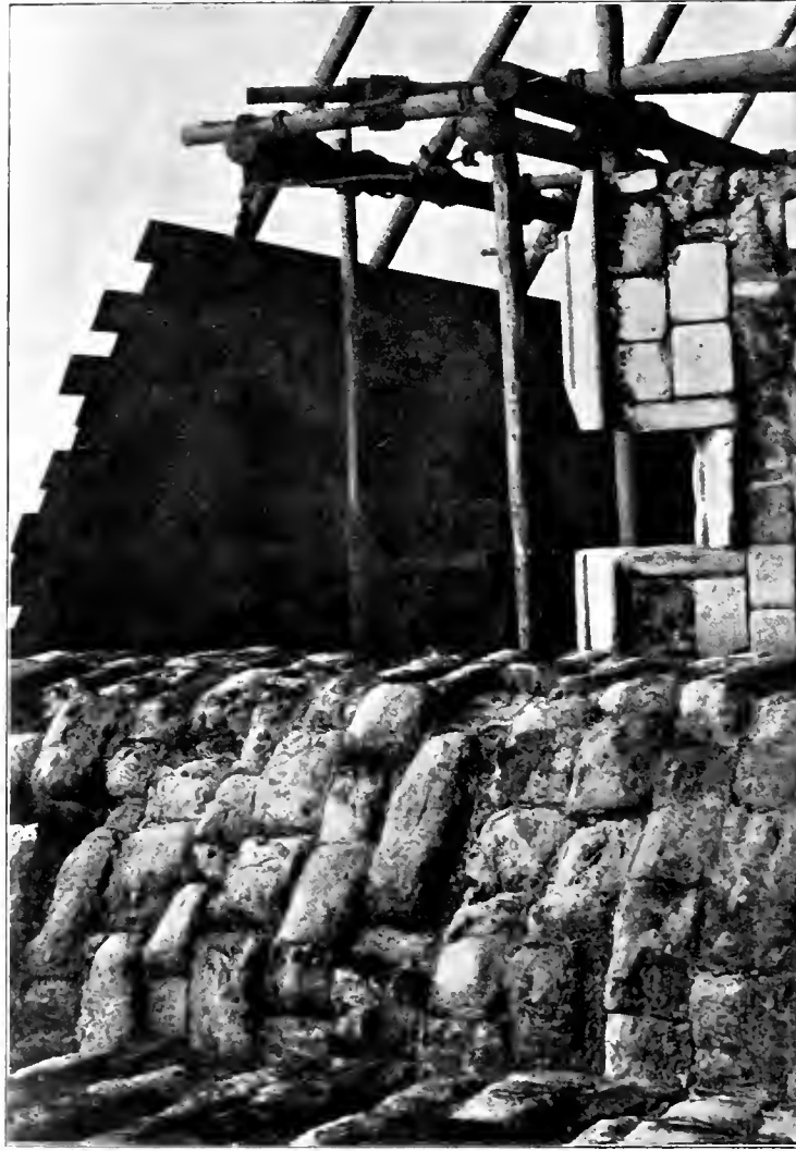
Stonework of Turret and North Aisle Battlement showing a previous restoration.
