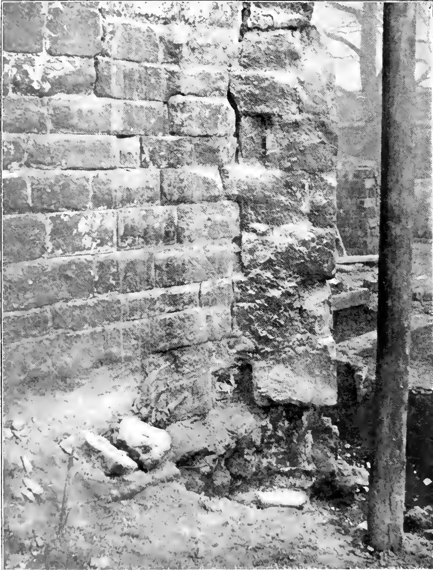
The South-East Buttress of the Chancel showing the fracture and settlement.
