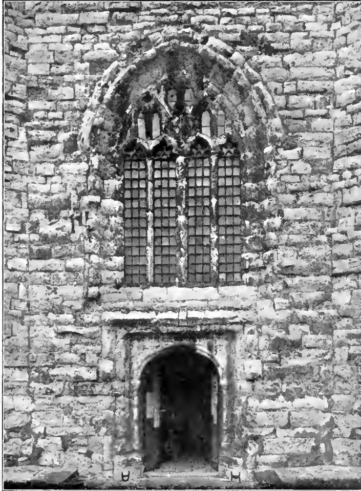
Detail of the West Doorway and Window, before the restoration, showing the decayed condition of the work.
