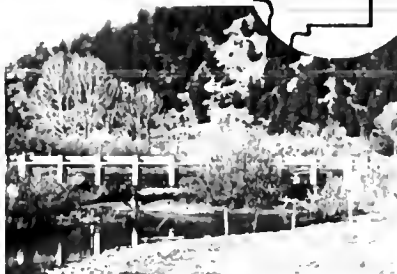
Before construction—note the split channel and how it widens the total area under the bridge.
