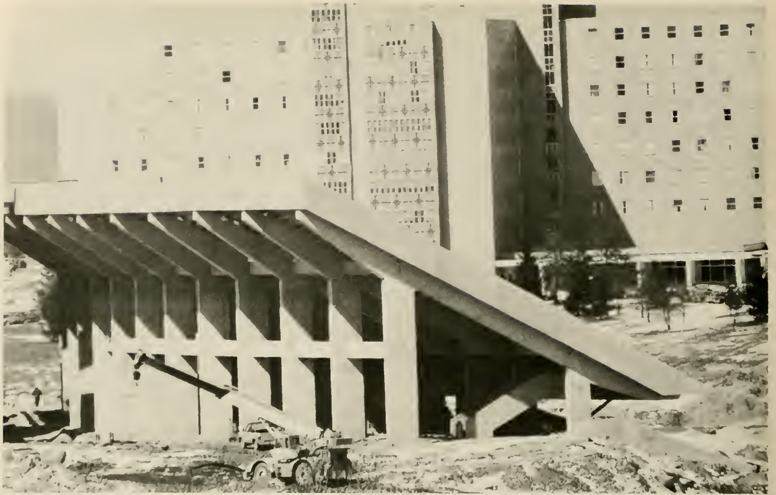
A mild winter permits the construction of the new stadium to continue.
