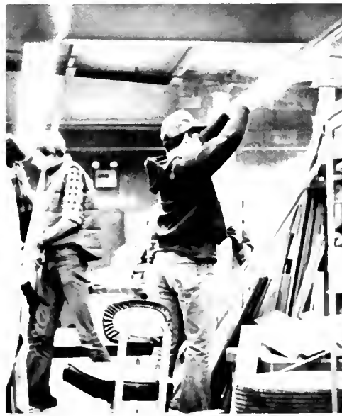
Jack Dever does some repair work on the PAC building for the organization
