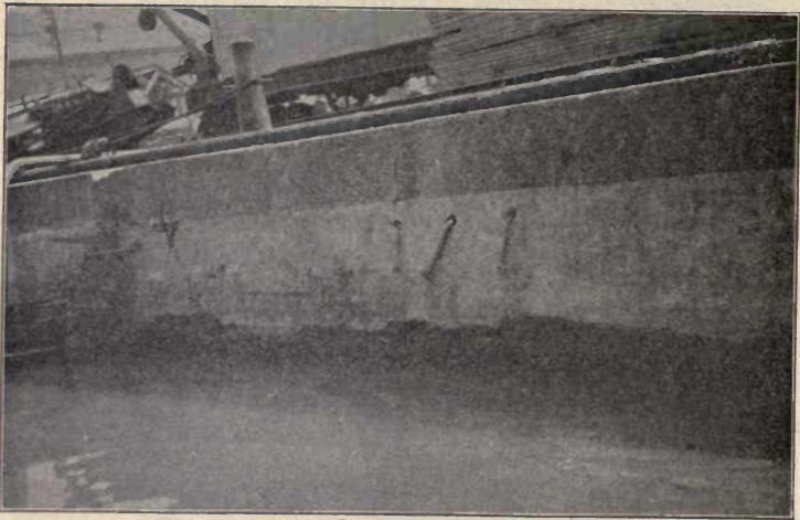
FIG. 244.—DISINTEGRATION OF CONCRETE THROUGH THE ACTION OF SALT WATER.
