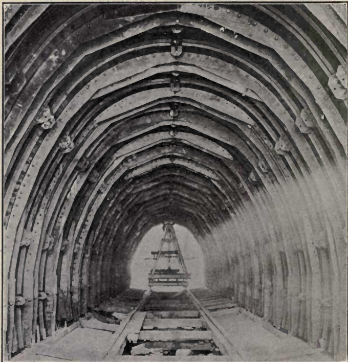
FIG. 24.—CUT-AND-COVER AQUEDUCT (CATSKILL), SHOWING INTERIOR OF STEEL FORMS FOR CONCRETE CAR FOR MOVING FORMS IN BACKGROUND.
