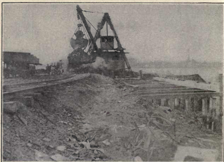
FIG. 159.—UNLOADING MACHINE, RIKER'S ISLAND, NEW YORK.
