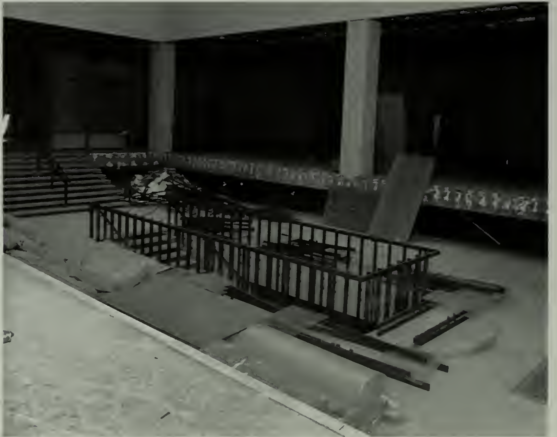
Renovation of the Marquand-Mather Court, The Art Museum, Princeton University. (a) Before renovation; (b) during renovation in 1989; (c) following completion of the new space. (Photos: [a and b] Clem Fiori; [c] William N. Taylor)
