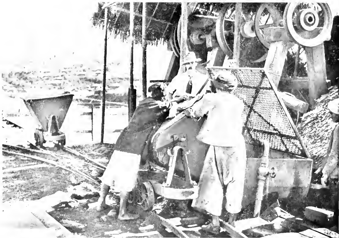
FIGURE 9. The trucks with locked covers. The contents of one are being tipped into the pulsator.
