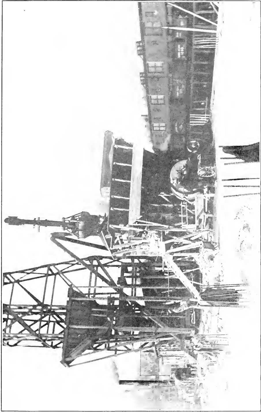
I. C. R. Halifax Terminals—Concrete mixing plant.
