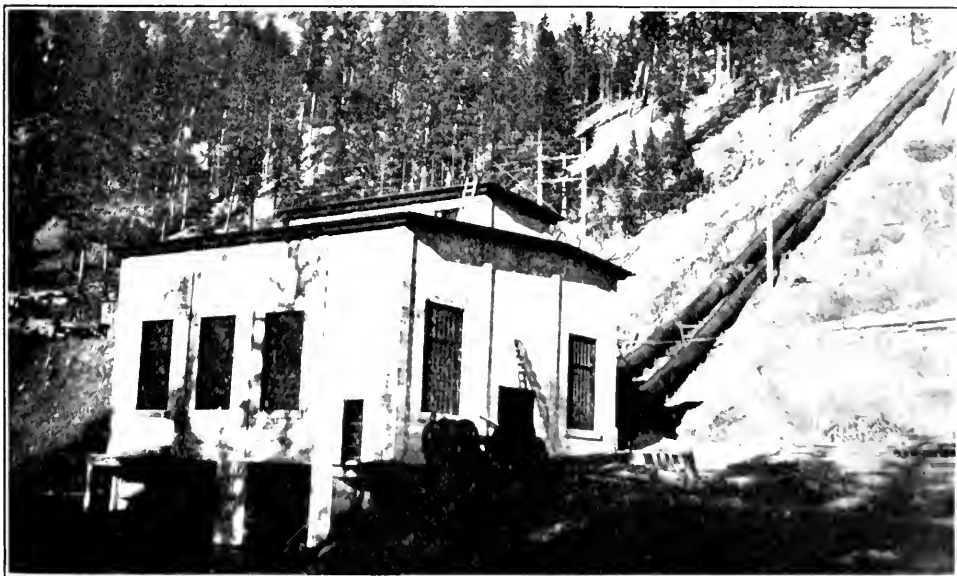
Exterior Barriere Hydro Electric Power House. Municipal plant for City of Kamloops, British Columbia.
