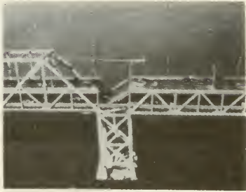
The San Francisco-Oakland Bay Bridge was damaged in the 1989 Loma Prieta earthquake
