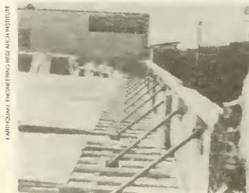
Bracing parapets can reduce damage and injuries
