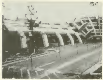
The 1994 Northridge, California, earthquake caused extensive damage to this parking garage
